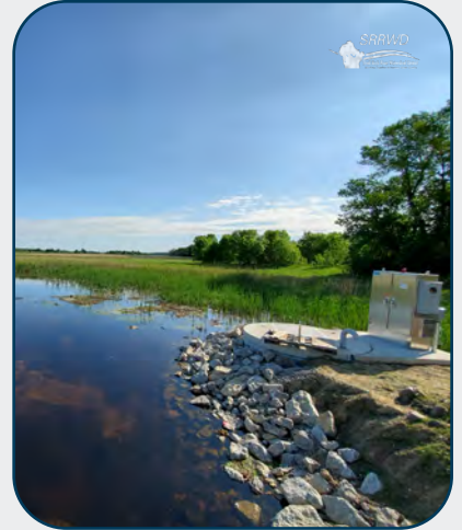
Upper Twin pump station
