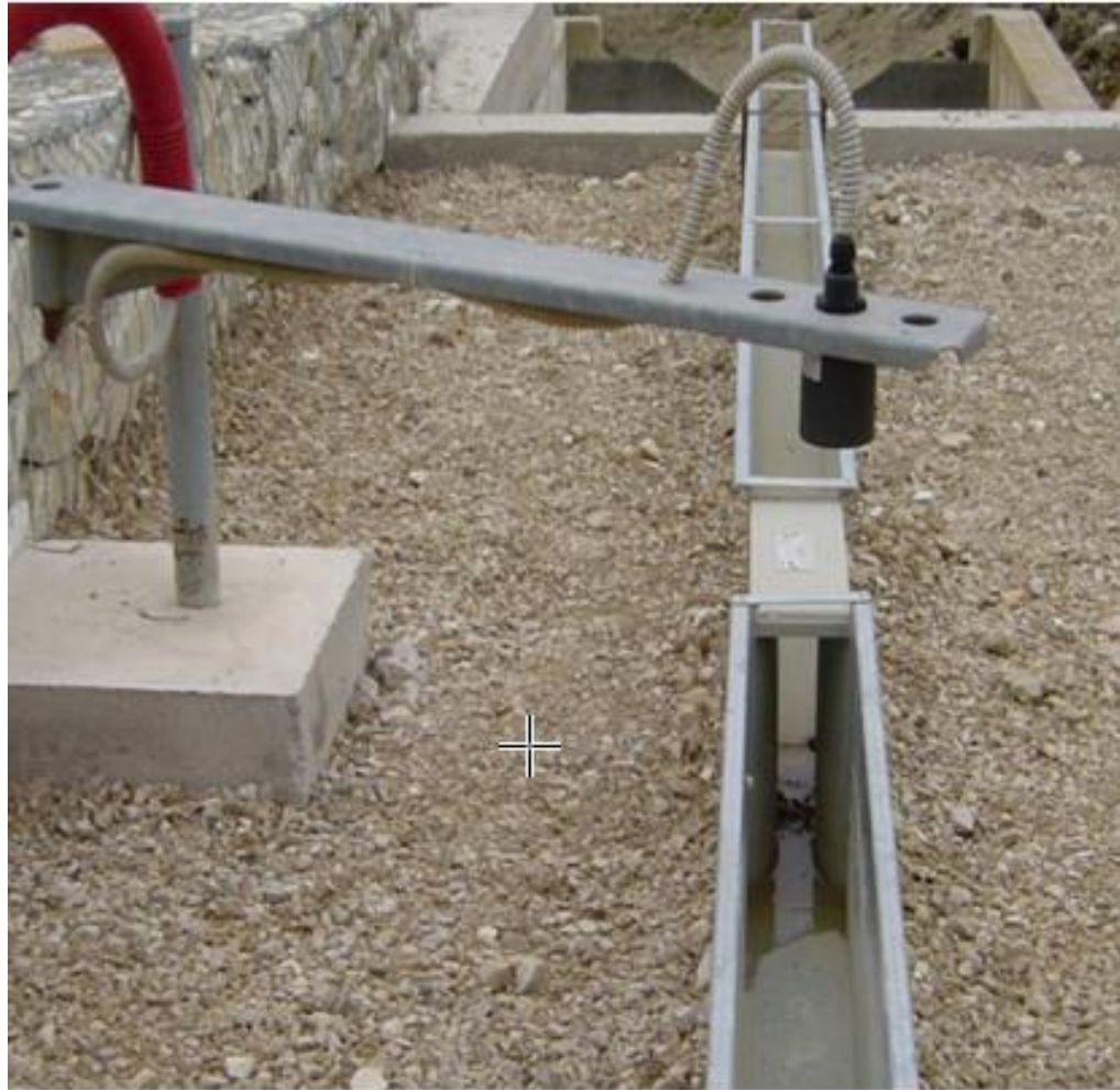
Fig. 4. View of the Venturi flume installed in the SPA1 measurement channel
