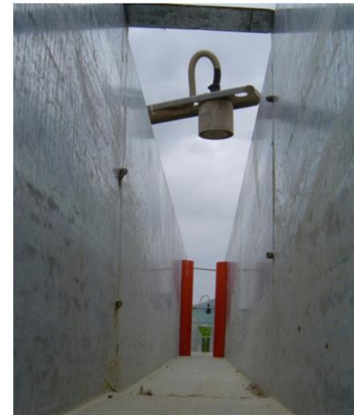
Fig. 3. View of the SMBF flowmeter installed in the SPA1 measurement channel
