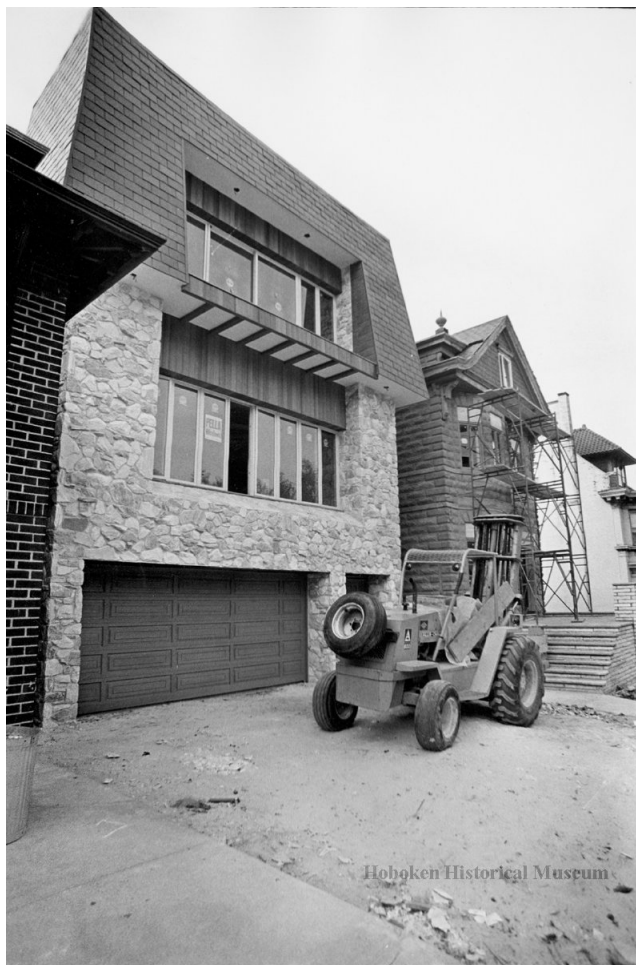
Figure 22. Photograph in the Hoboken Historical Museum's collections depicting the construction of 914 Castle Point Terrace (Property ID 134222107) in the late 1960s or early 1970s (Source: Hoboken Historical Museum).
