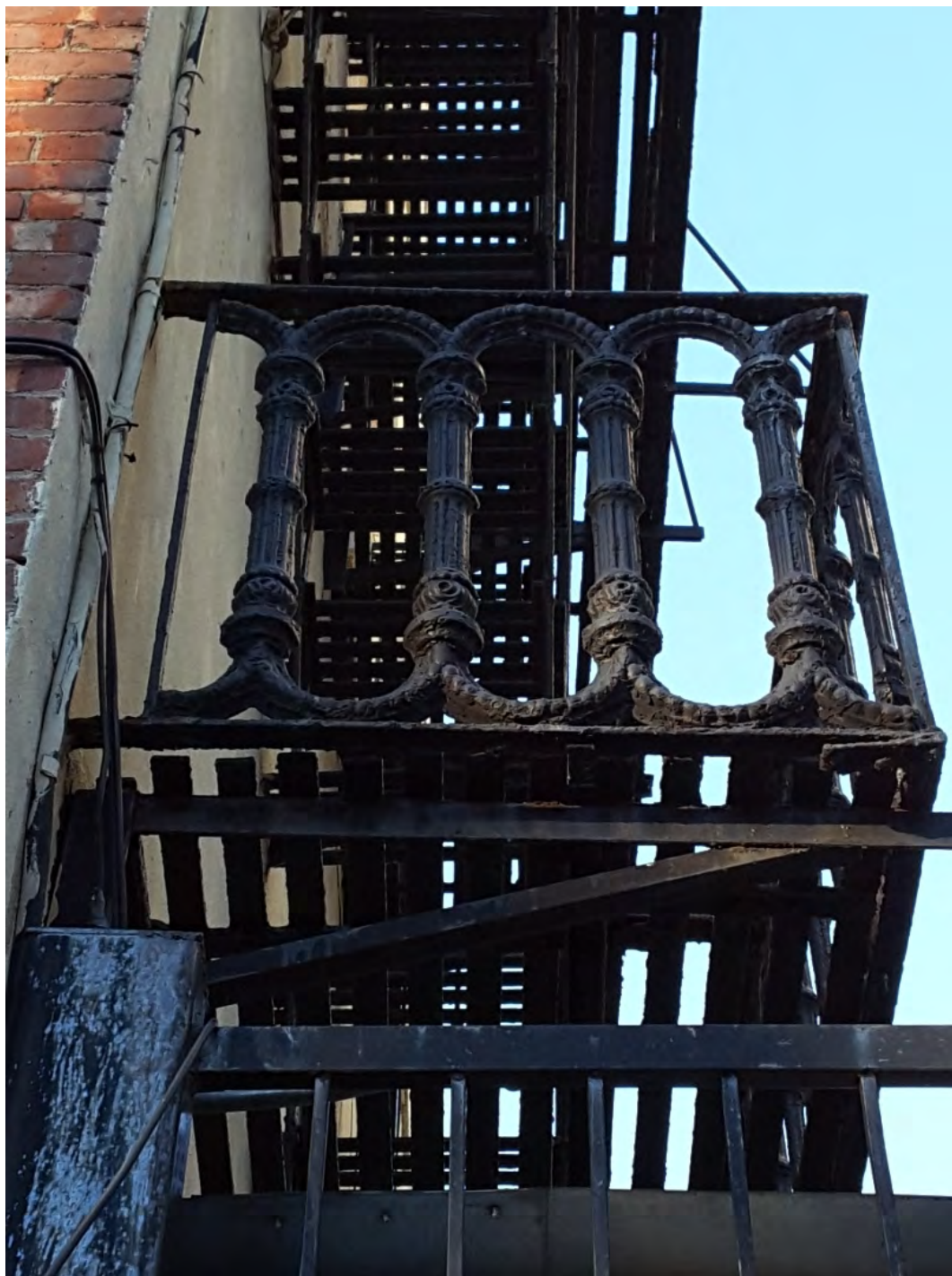
Photograph 5. Detail view of the cast iron fire escape on the east elevation of the Odenheimer House.
