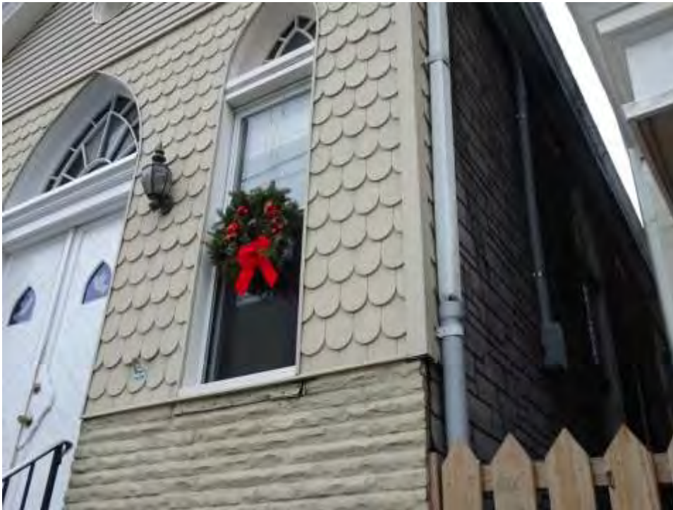
Photograph 2. The chapel is clad in a variety of replacement materials. Detail view south.
