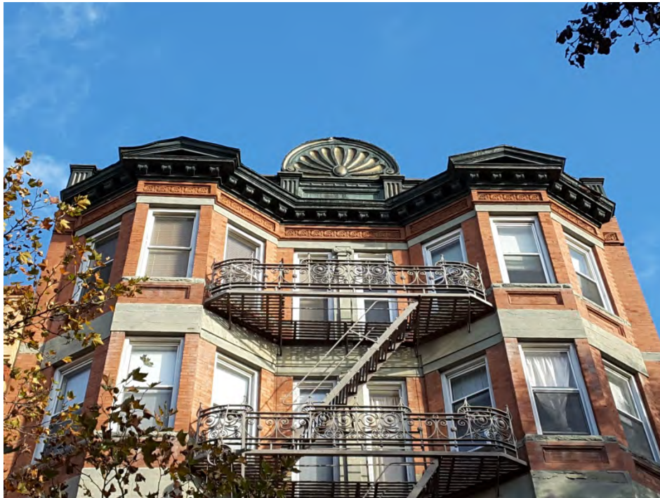
Photograph 5. Detail view of the upper floors and cornice of the Marguerite apartment building. Note the terra cotta tiles.
