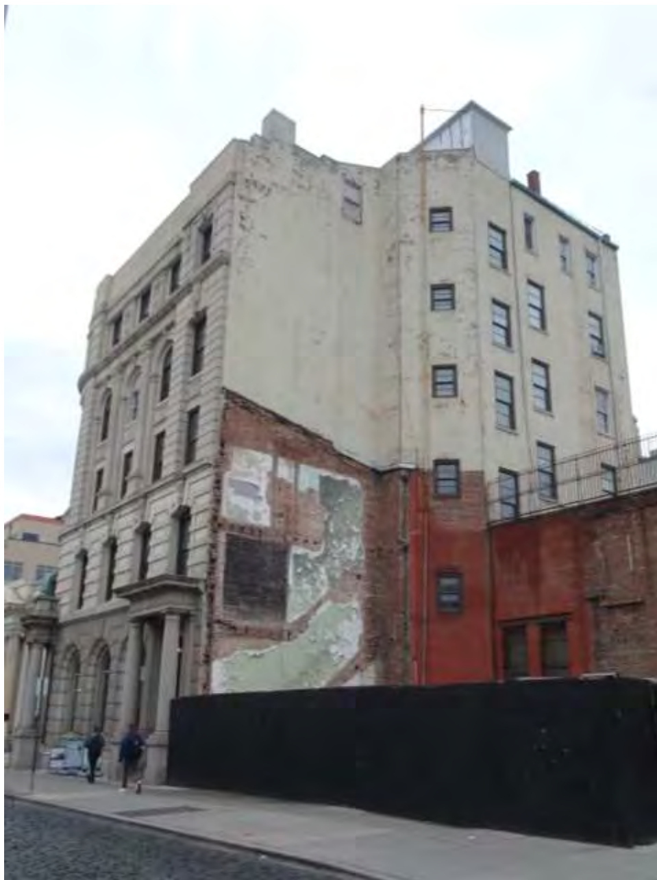
Photograph 5. View southeast of the northern elevation. Until 2017, the northern elevation was directly adjacent to a three-story brick structure that predated the Hudson Trust Building.
