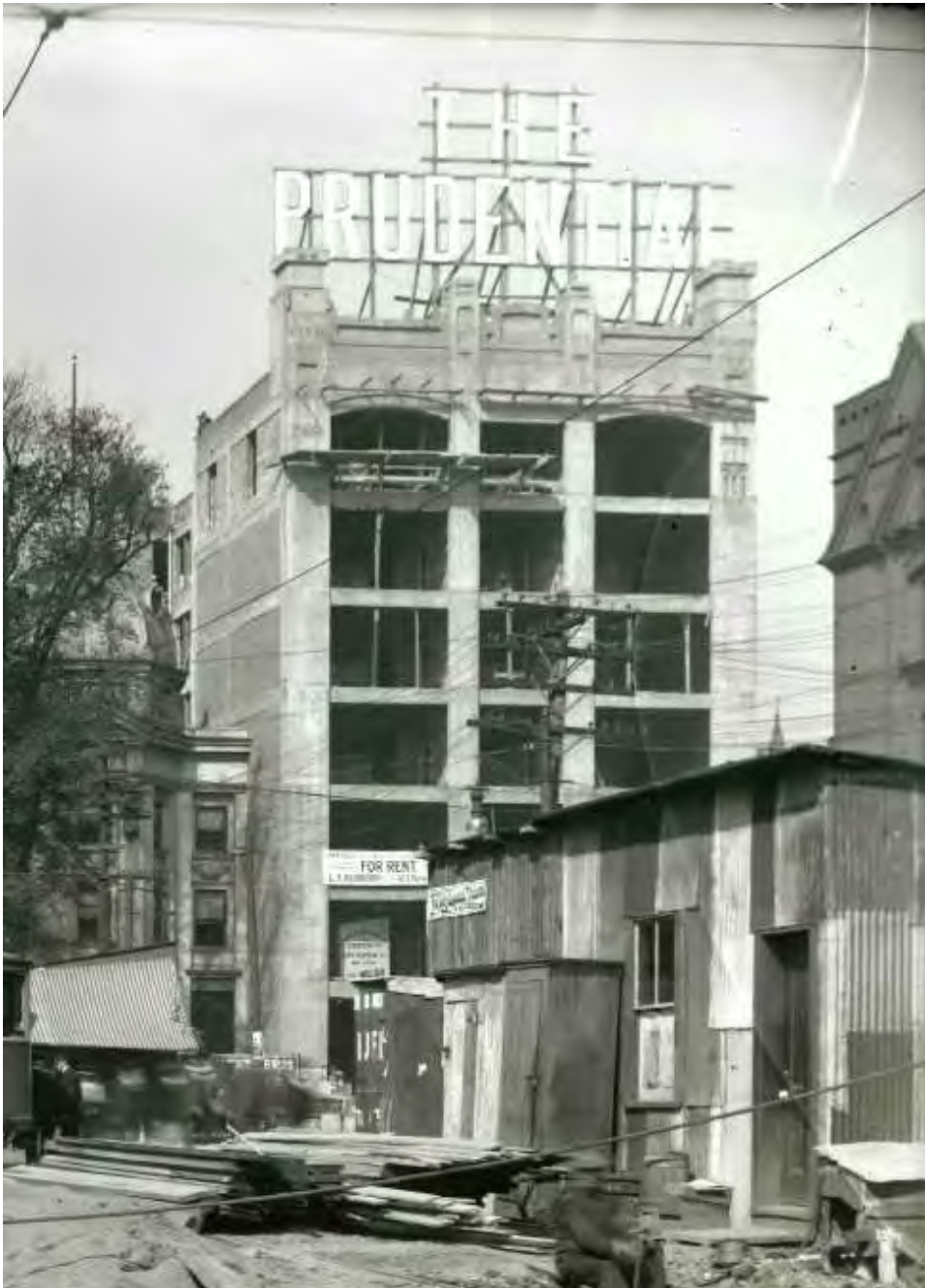
Figure 3. View of the Terminal Building while under construction, ca. 1909, view north west from Hudson Place. Note the “The Prudential” signage on the roof, showing the early stages of the installation of the iconic Rock of Gibraltar sign (Source: Hoboken Historical Museum 1 ).
