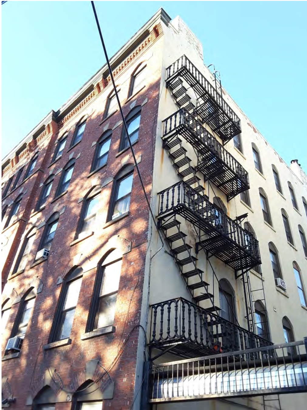
Photograph 3. View of the southeast corner of the Odenheimer House building, depicting the cast iron fire escape on the east elevation of the structure.
