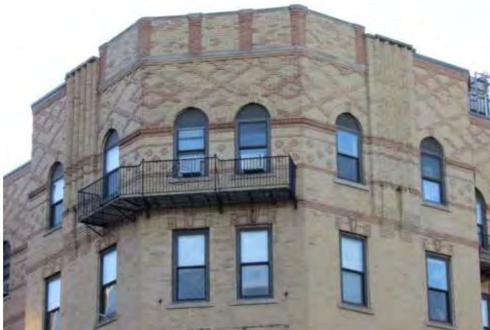
Photograph 2. Close-up view of the parapet at the north corner of the complex, view southeast.
