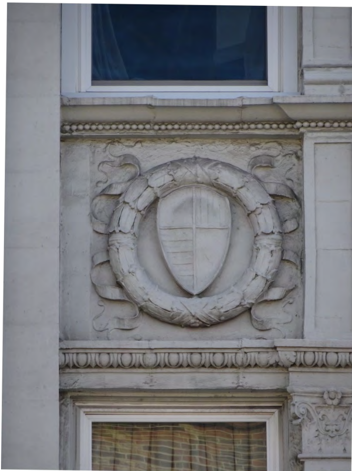
Photograph 6. Detail view of the faux-historic ca.1985 terra cotta detailing on the primary elevation of the building.
