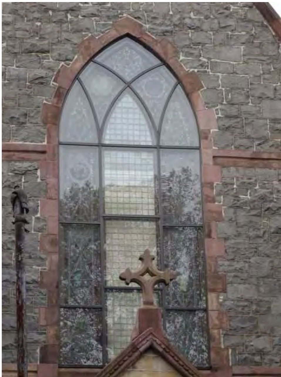
Photograph 6. Detail of the main stained glass window on the primary façade, view west.
