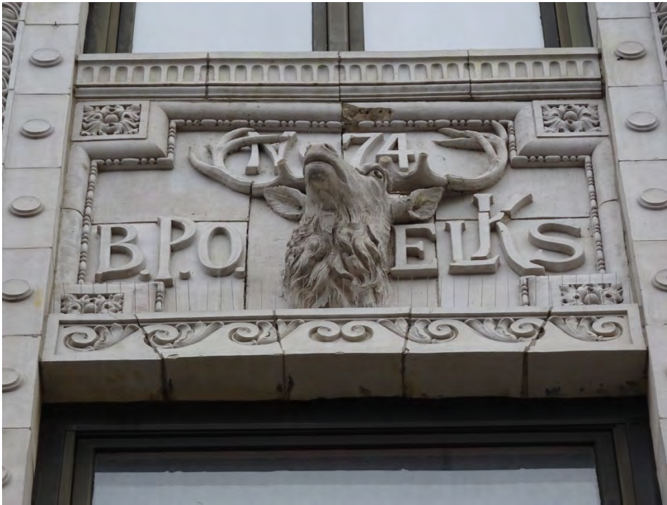
Photograph 5. Detail view of terracotta details between windows on the facade, view east.
