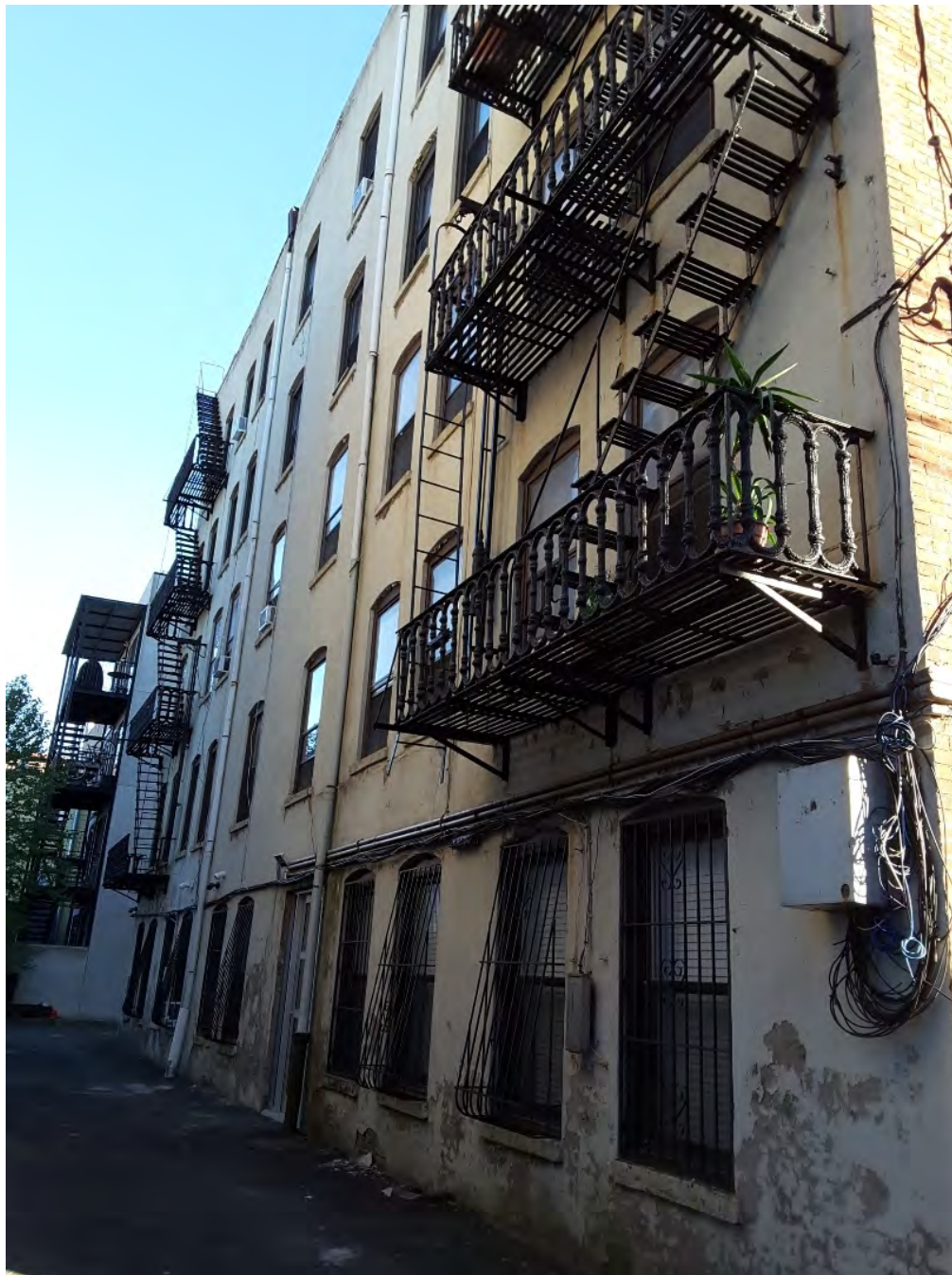
Photograph 4. View of the rear (north) elevation of the Odenheimer House, showing the rear entry and the twin cast iron fire escapes.
