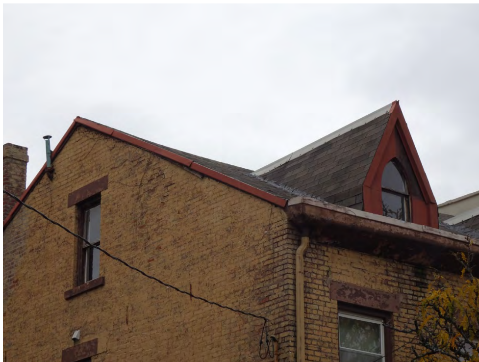
Photograph 7. Detail view of the roof and pointed dormers on the rectory building, view northwest.
