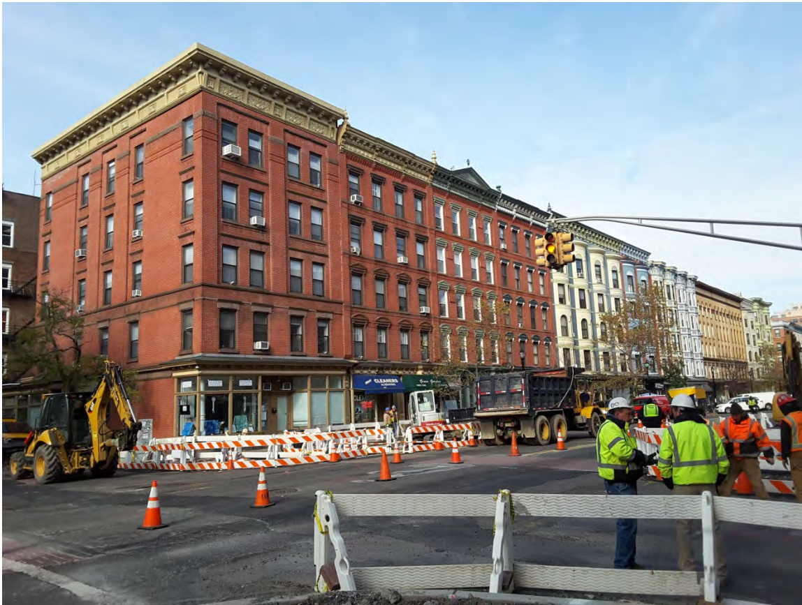
Photograph 4. Construction activities along Washington Street. View of the northwest corner of the intersection of Washington and Twelfth Streets looking northwest.
