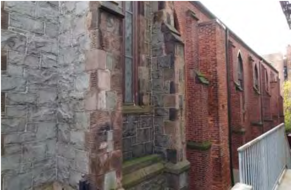
Photograph 2. The north elevation drops down a story from street level, view southwest.
