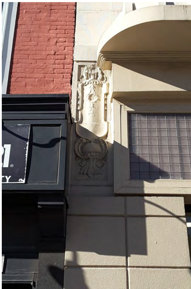
Photograph 4. Detail view of terra cotta ornamentation on the Washington Street façade of the Geismar-Meyer Co. Department Store building.
