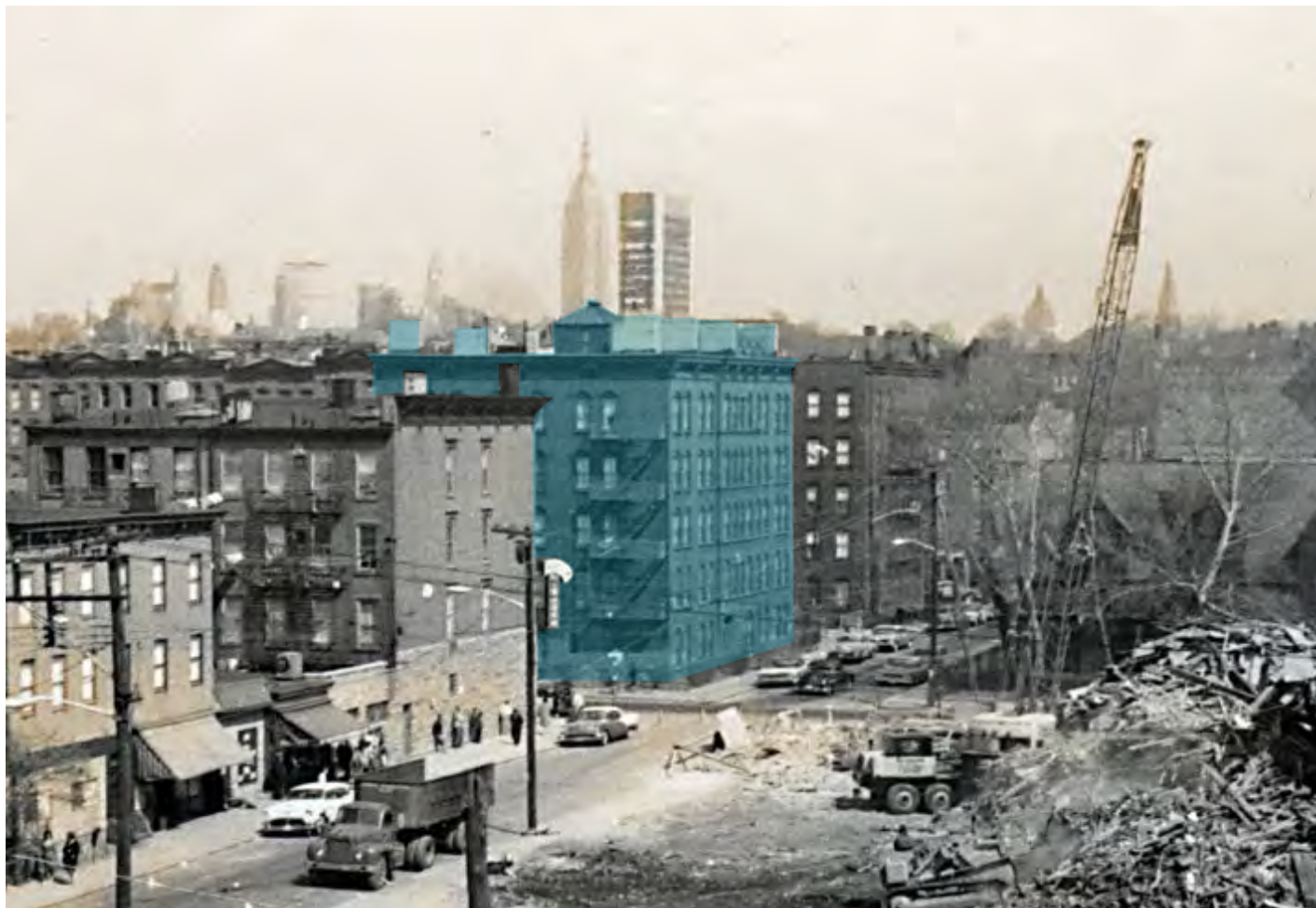
Figure 7. The Odenheimer House (highlighted) in a ca. 1963 photograph (Source: Hoboken Historical Museum).
