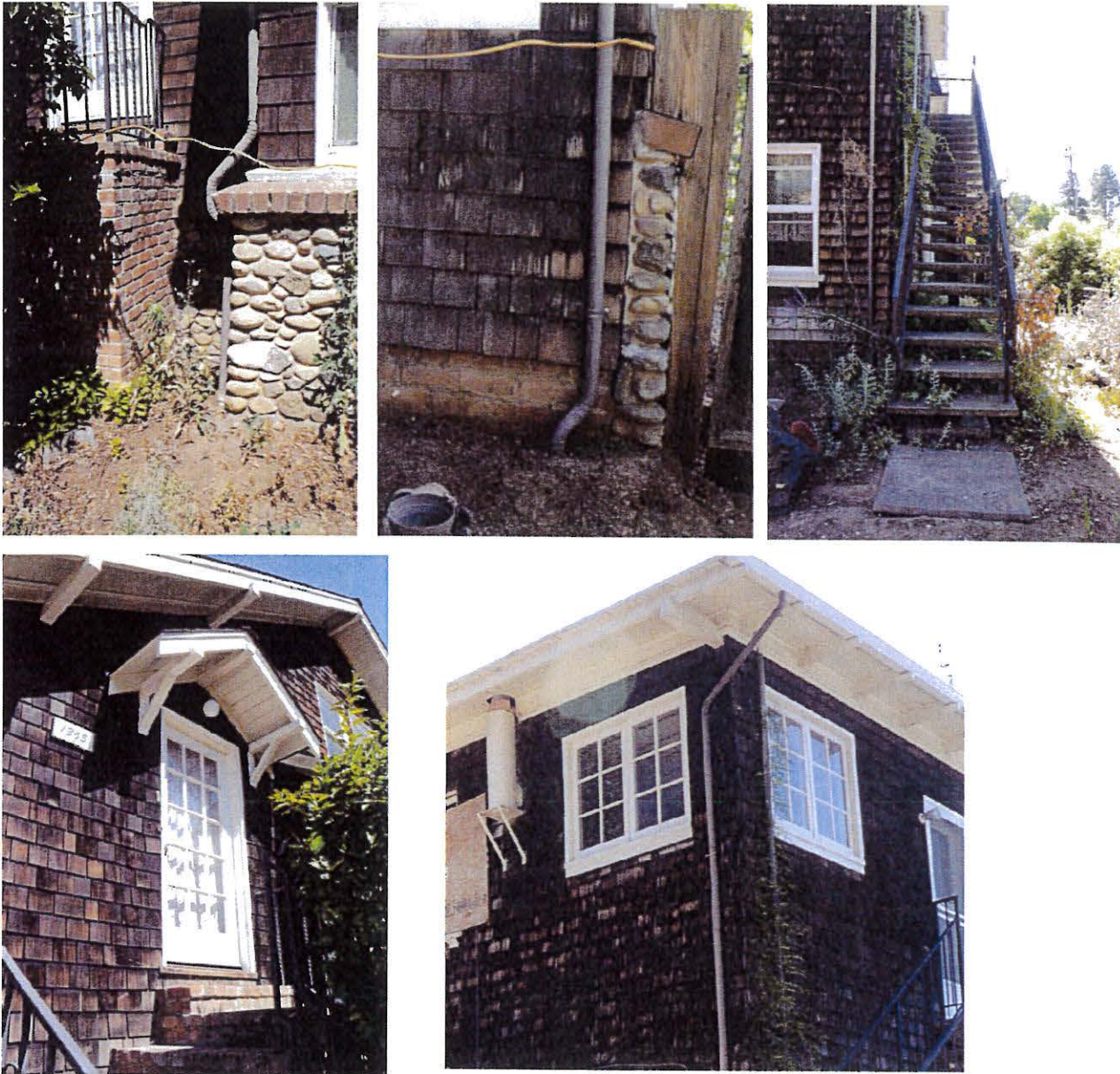
Image 24-28. Alterations to the house: brick stair (top left); applied river rock finish and brick sill course (top center); the concrete plank stair and metal railing (top right); stair entry door; and east end of the building has a low-pitched roof and corner windows reminiscent of 1930s and 1940s architecture.
