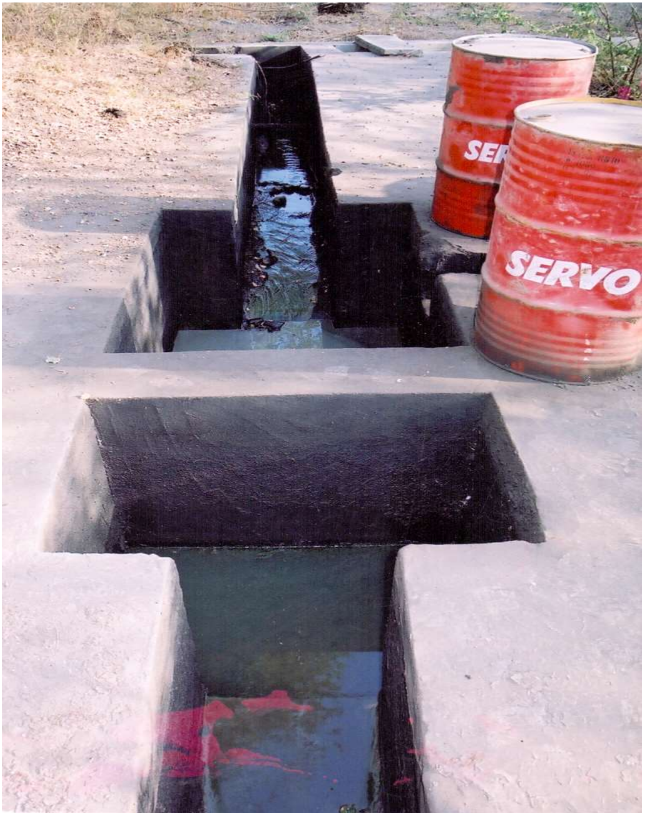
Oil & Grease trap photo
