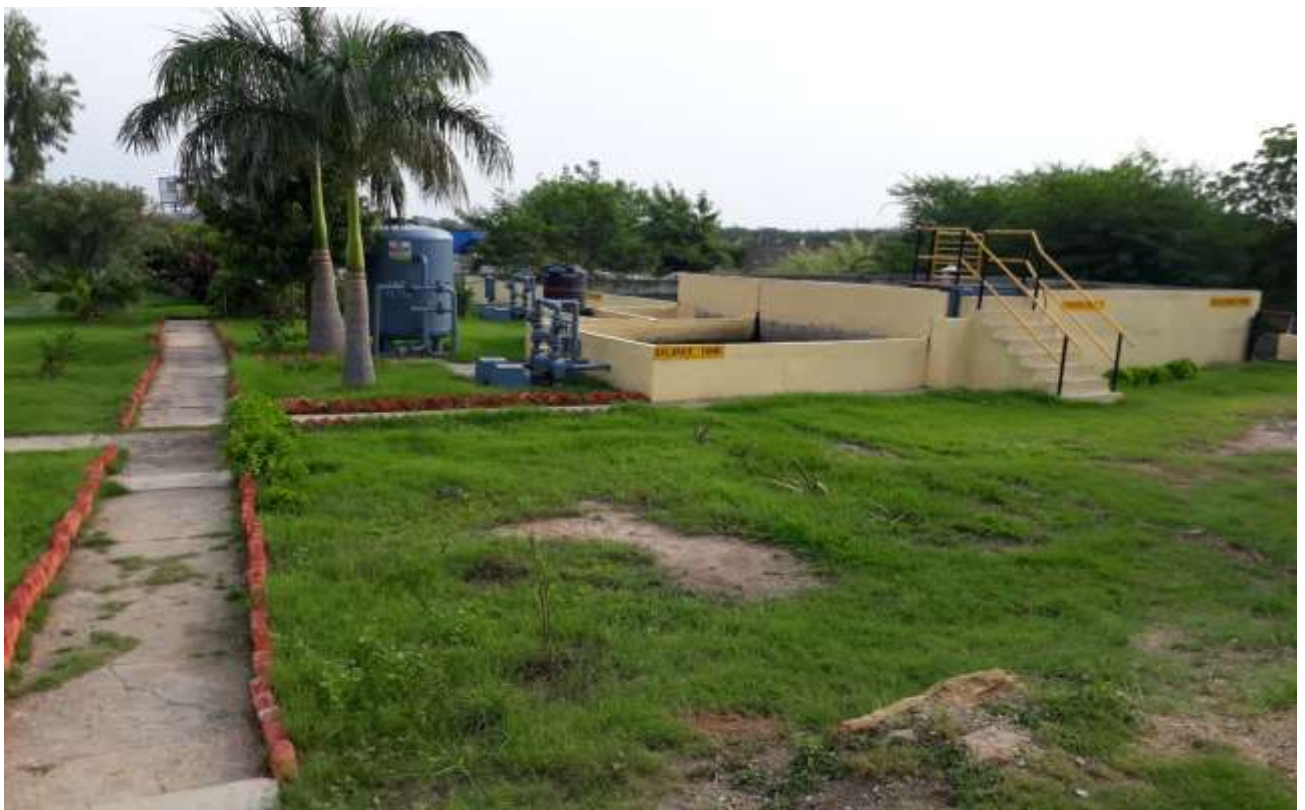
STP (300KLD) in plant premises
