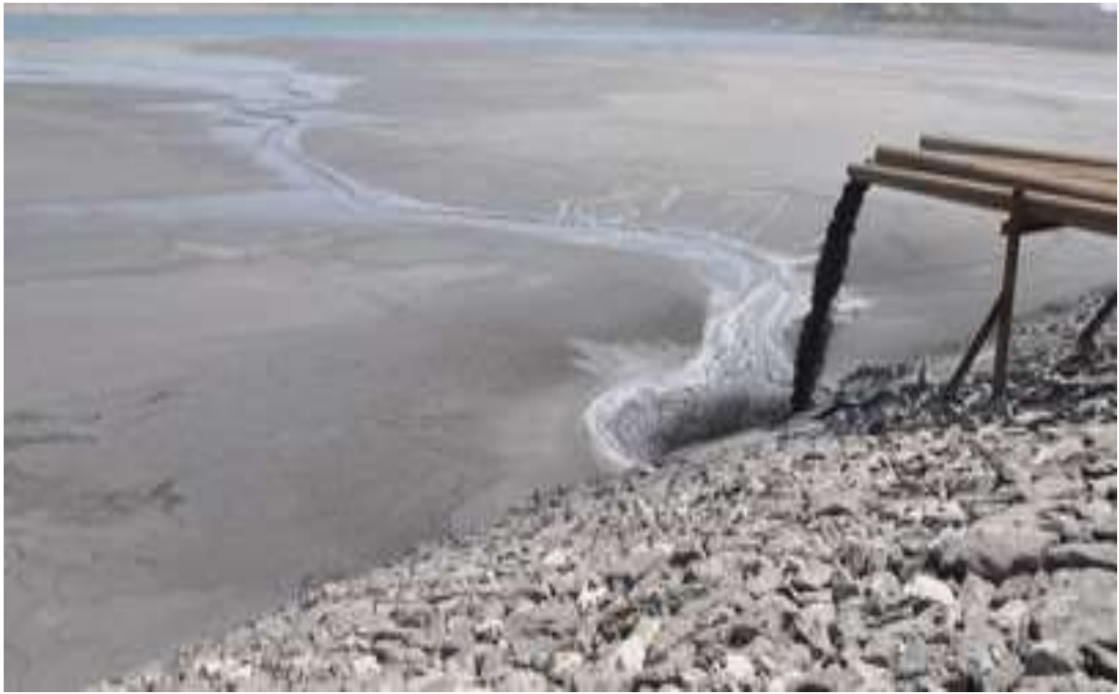
Tailing close pipe line
