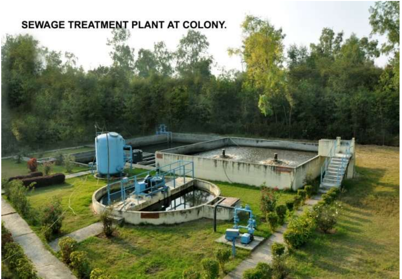
STP (425KLD) in plant premises
