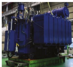
Figure 2 | Synthetic ester oil transformer - 33kV 60MVA
