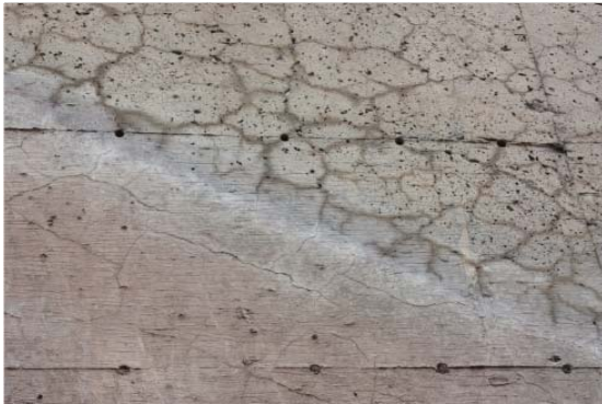
Figure 3.2. A&B. Map-cracking in wing walls (exposed elements) of bridge structures affected by ASR. C. Cracking in the column and the exposed portion of a beam affected by ASR. D&E. Cracking in the exposed portion (above ground) of the wing wall of a bridge structure affected by ASR; the wing wall has been excavated before being demolished. The lower ground portion shows limited cracking; discoloration occurs around the cracks above ground (E).
