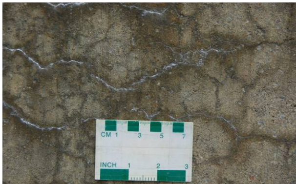
Figure 3.6. A. Pop-out created by the expansion of a frost-susceptible porous coarse aggregate particle (leached chert). B. ASR-induced pop-out in a concrete pavement incorporating highly-reactive aggregates; also noted pattern cracking. C. Efflorescence and exudations of alkali-silica gel at the surface of the concrete foundation of 25-year-old highway bridge affected by ASR. D. Efflorescence and exudations of alkali-silica gel at the surface of a small concrete monument affected by ASR. E. Surface discoloration and exudation associated with cracks.
