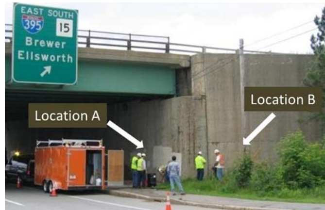
Figure 8.4. Photograph of bridge in Bangor, Maine. Location A is sheltered by the bridge deck, whereas Location B is exposed directly to precipitation. Sampling of concrete cores from each location showed strong correlation between moisture availability and ASR-induced expansion and cracking.
