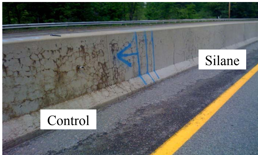
Figure 8.10. Reduction in Cracking of Highway Barriers in Massachusetts, after Application of Silane (FHWA Project DTFH61-06-D-00035)
