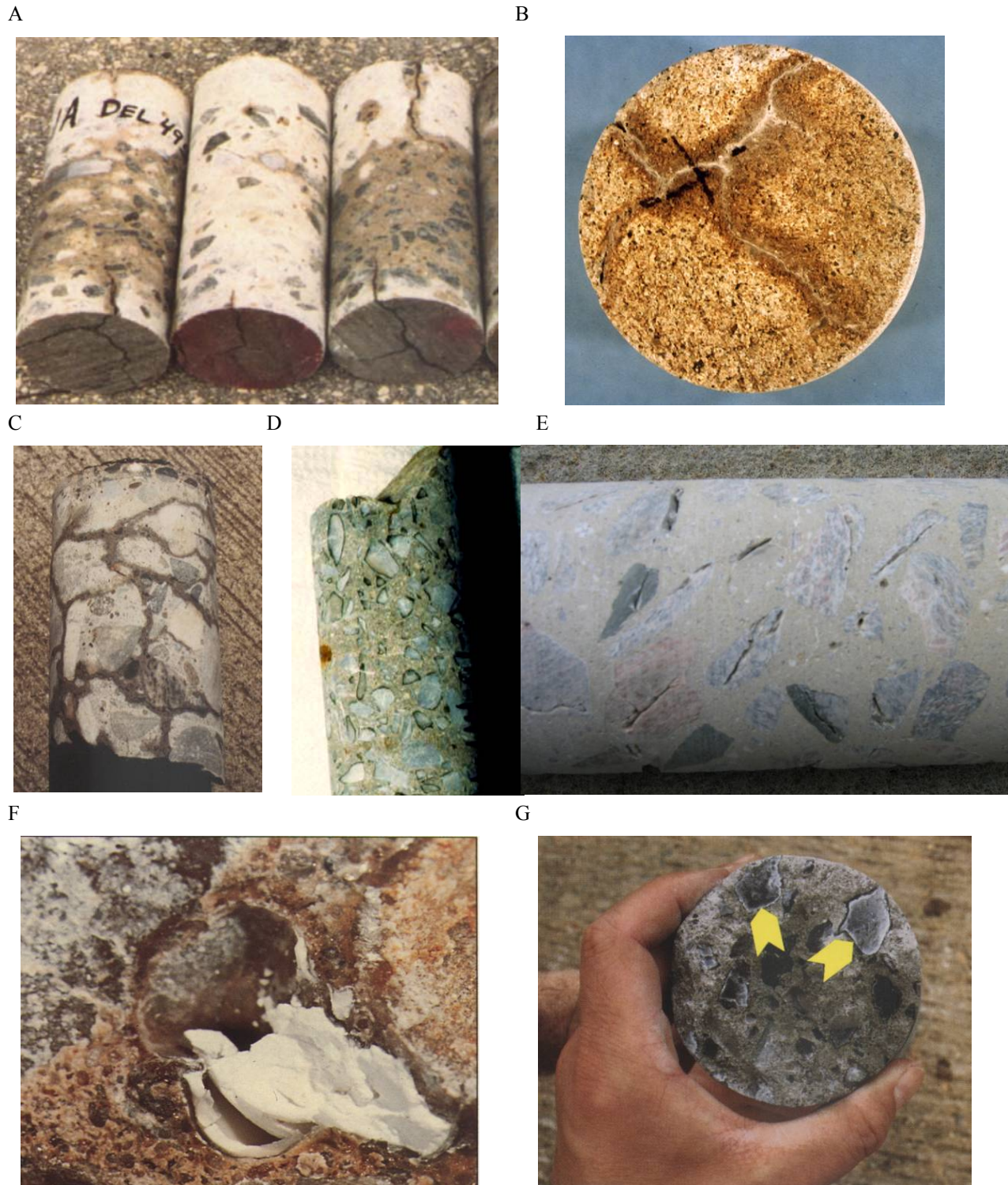
Figure 7.5. Macroscopic observations on cores (as received condition). A. Cores extracted from a concrete pavement affected by ASR and showing macrocracks penetrating from the upper and lower parts of the pavement. B. Gel staining surrounding cracks and gel exudations at the surface of a core extracted from a sidewalk section affected by ASR. C. Fine cracking pattern showing up after re-wetting of the core. D. Dark rim surrounding reactive aggregate particles. E. Macrocracks in reactive coarse aggregate particles. F. Deposits of alkali-silica gel in a void on core surface. G. Deposits of alkali-silica reaction products on the broken surface of a core extracted from a highway bridge structures affected by ASR.
