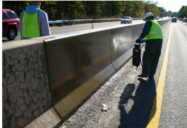
Figure 8.6. Photograph Showing Topical Application of 40%-Silane Solution (solvent-based) to ASR-Affected Highway Barrier in Massachusetts (part of FHWA Project DTFH61-02-C-00097)
