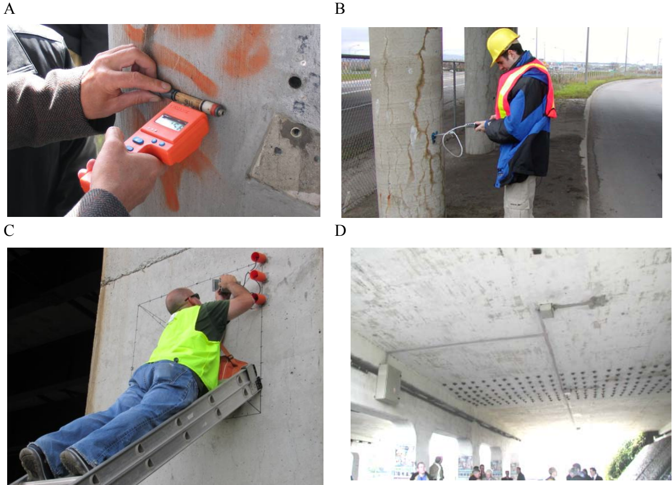
Figure 7.11. In-situ measurements of humidity in concrete. A. Wooden-stick method. B-C. Portable humidity probes. D. Automatic in-situ monitoring of temperature, humidity and expansion (vibrating wire) in a bridge deck affected by ASR (Siemes and Gulikers 2000).
