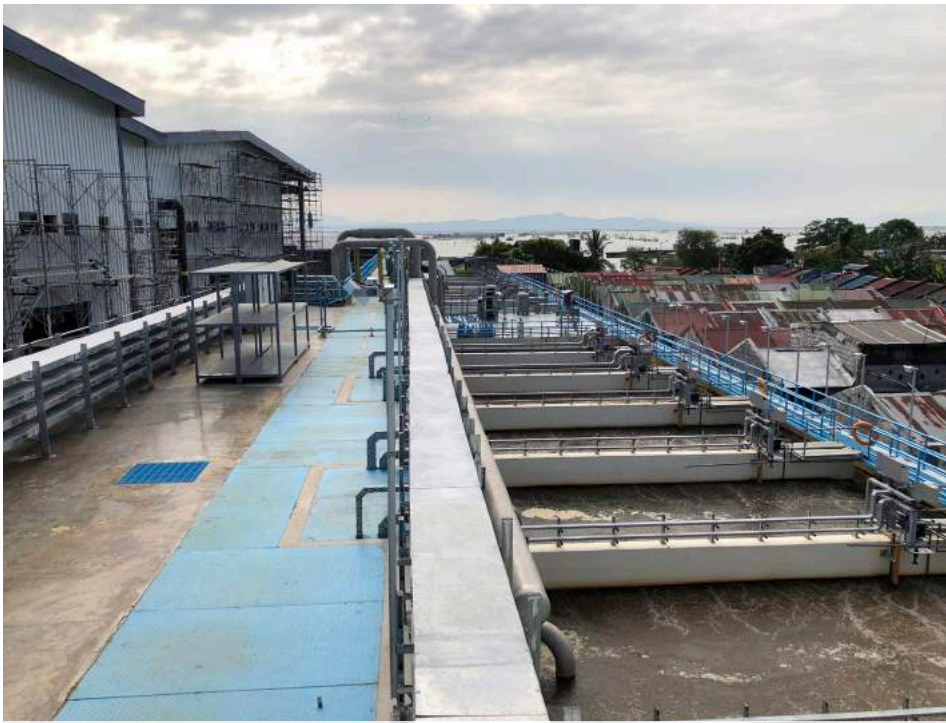
The huge Putatan water treatment plant helped Manila secure its water supply in the face of a savage drought
