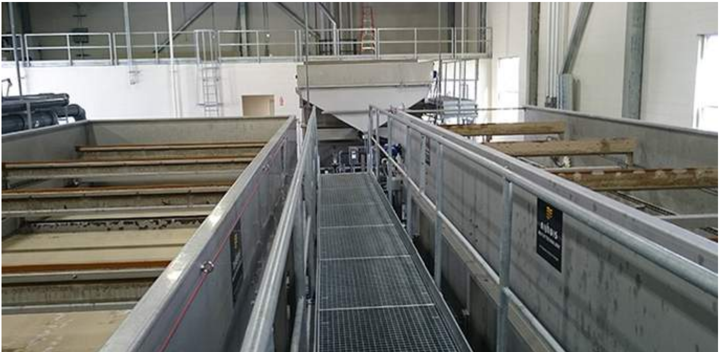
Nijhuis found new uses for industrial treatment technologies that saw its capabilities soar over the course of the year
