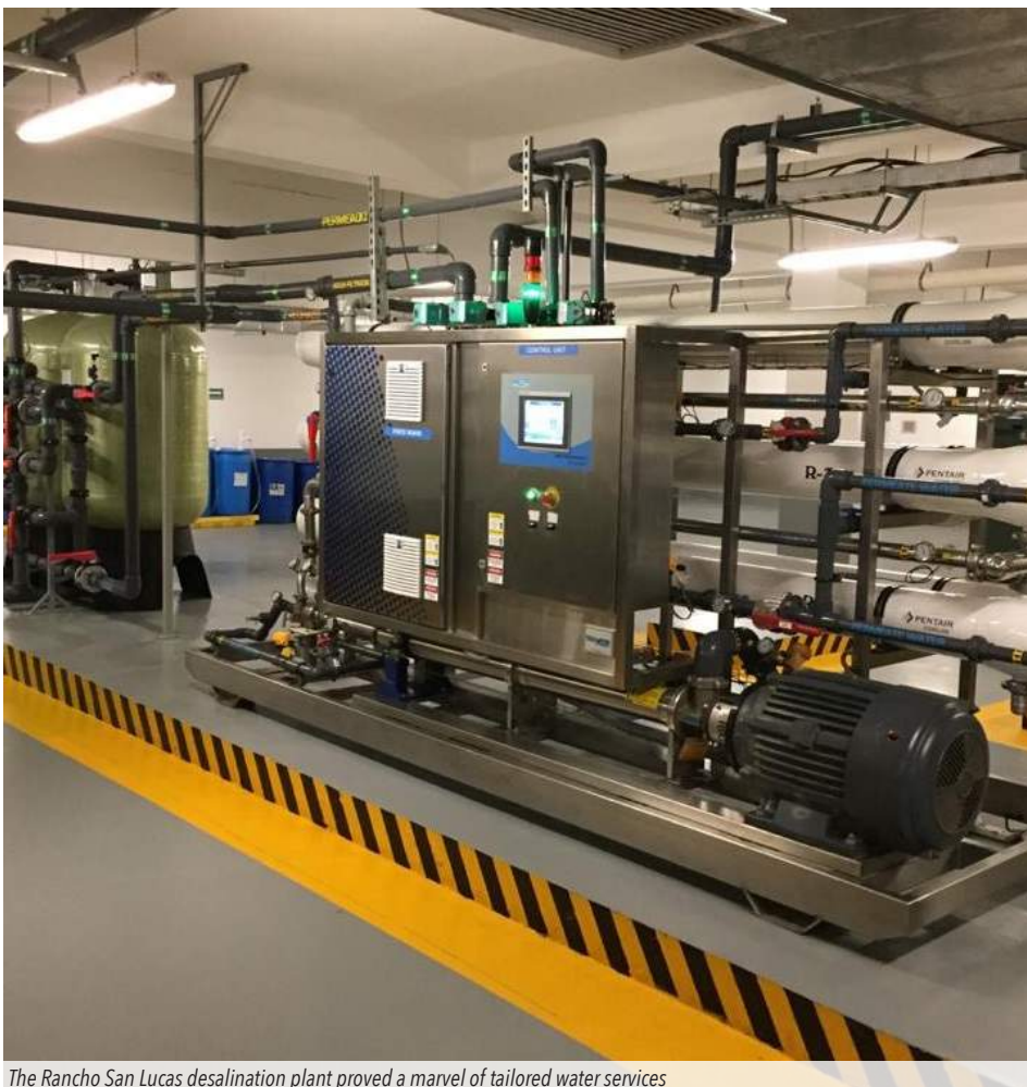
The Rancho San Lucas desalination plant proved a marvel of tailored water services
