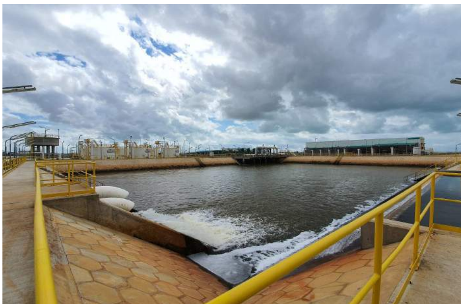
The Petronas IETP in Malaysia is one of the largest of its type in the world and treats an array of nasty effluents
