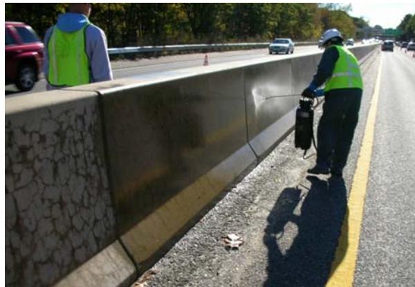
Figure 8.6. Photograph Showing Topical Application of 40%-Silane Solution (solvent-based) to ASR-Affected Highway Barrier in Massachusetts (part of FHWA Project DTFH61-02-C-00097)
