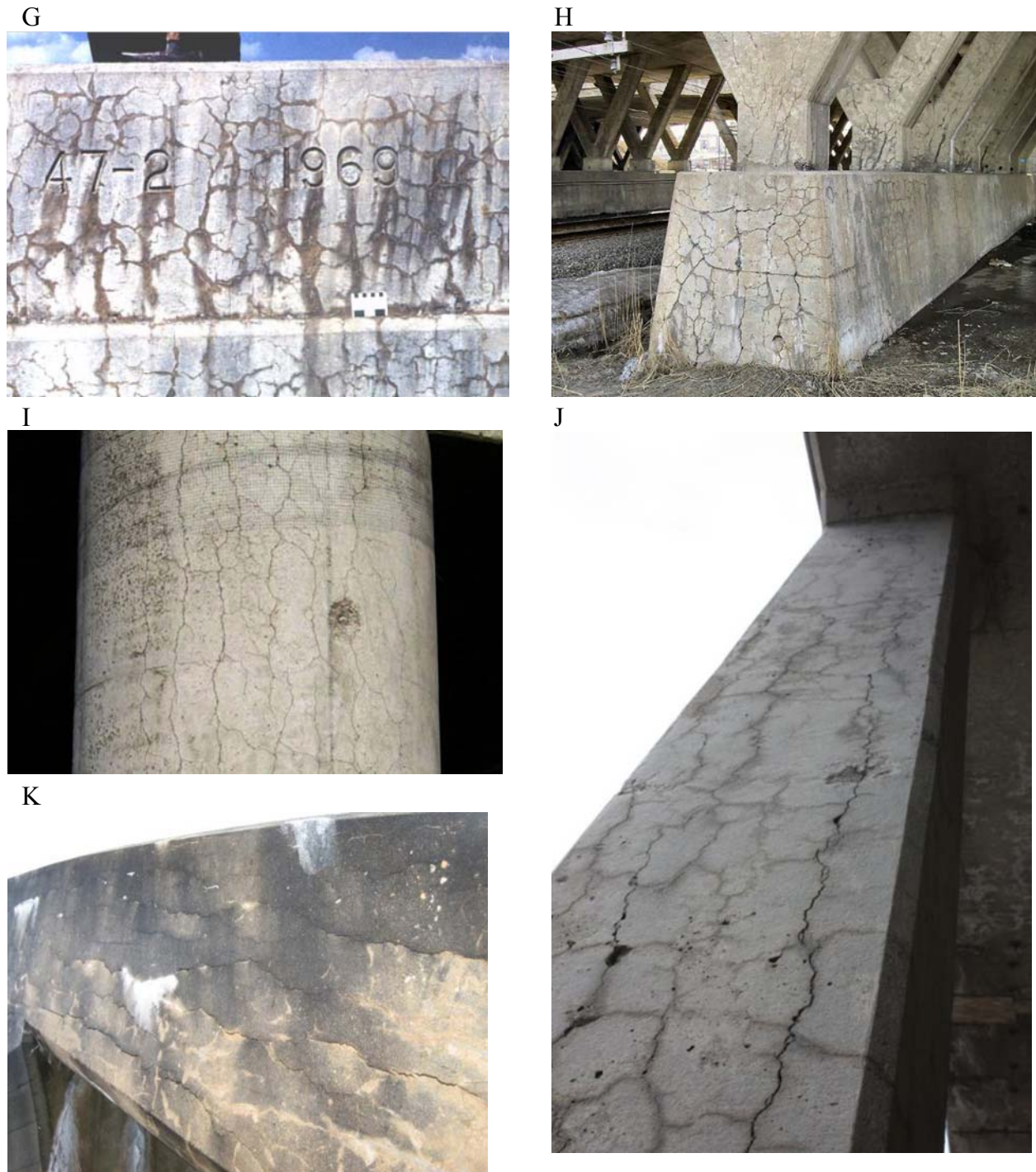
Figure 7.2 (cont'd). ASR-related defects in bridge elements and severity assessment. G. Map cracking on a parapet wall (condition state 3); moderate gel exudations are also present, which give the impression of permanent dampness. H. Map cracking in massive column foundation block of a bridge structure (condition state 3). I. Aligned (vertical/longitudinal) cracking in reinforced concrete column (condition state 2). J. Severe (condition state 3) aligned (longitudinal) cracking connected by moderate map cracking in a reinforced concrete column. K. Aligned (longitudinal) cracking in the top chord of a reinforced concrete arch bridge (condition state 3 to 4).
