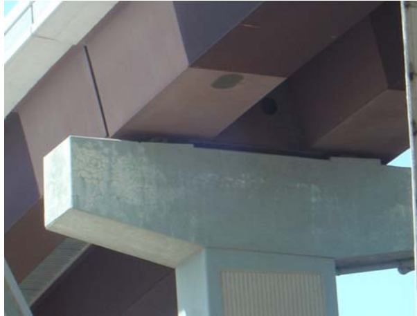
Figure 8.3. Photograph of bridge in Houston, Texas, illustrating effects of moisture availability on ASR-induced expansion and cracking. Only the exposed face of the bent cap (left side of photo) shows visual cracking, whereas the portions of the bent cap protected by the bridge deck show very little cracking.
