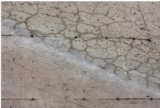
Figure 3.2. A&B. Map-cracking in wing walls (exposed elements) of bridge structures affected by ASR. C. Cracking in the column and the exposed portion of a beam affected by ASR. D&E. Cracking in the exposed portion (above ground) of the wing wall of a bridge structure affected by ASR; the wing wall has been excavated before being demolished. The lower ground portion shows limited cracking; discoloration occurs around the cracks above ground (E).
