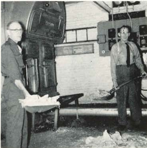
Day custodians, Charlie Fineran and Jim Thomas, keep the boiler room spic and span as they get rid of a saw dust pile.
