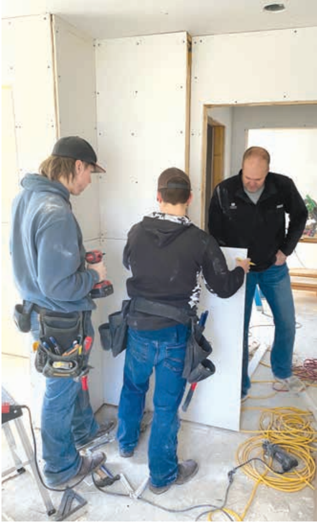
From right, instructor Tim Phillips observes, as DCTC students Joel Hyder and Porter Hensley secure, measure and cut drywall.
