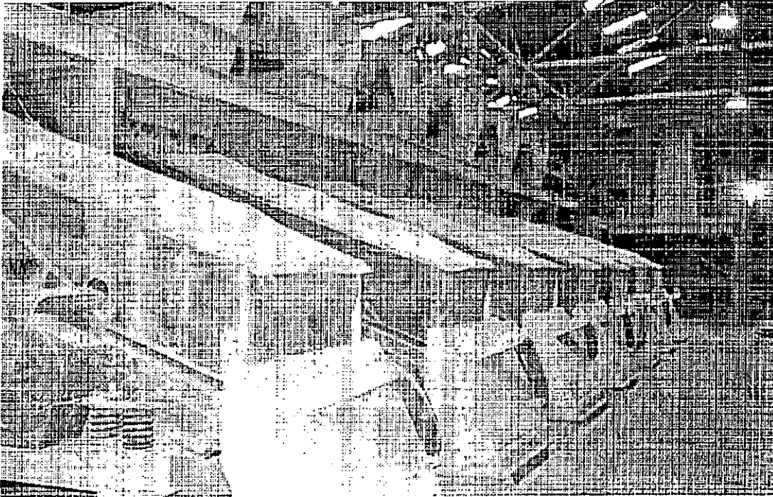
Figure 18. Plant 8 screens and hoods.
