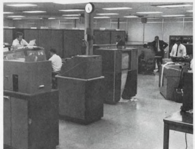
Layout of center must conform to predetermined pattern with one-third of an inch to avoid losses and cross talk in connecting cables. The method of redundancy through switching rather than by means of more equipment results in more wiring and cables than usual.
