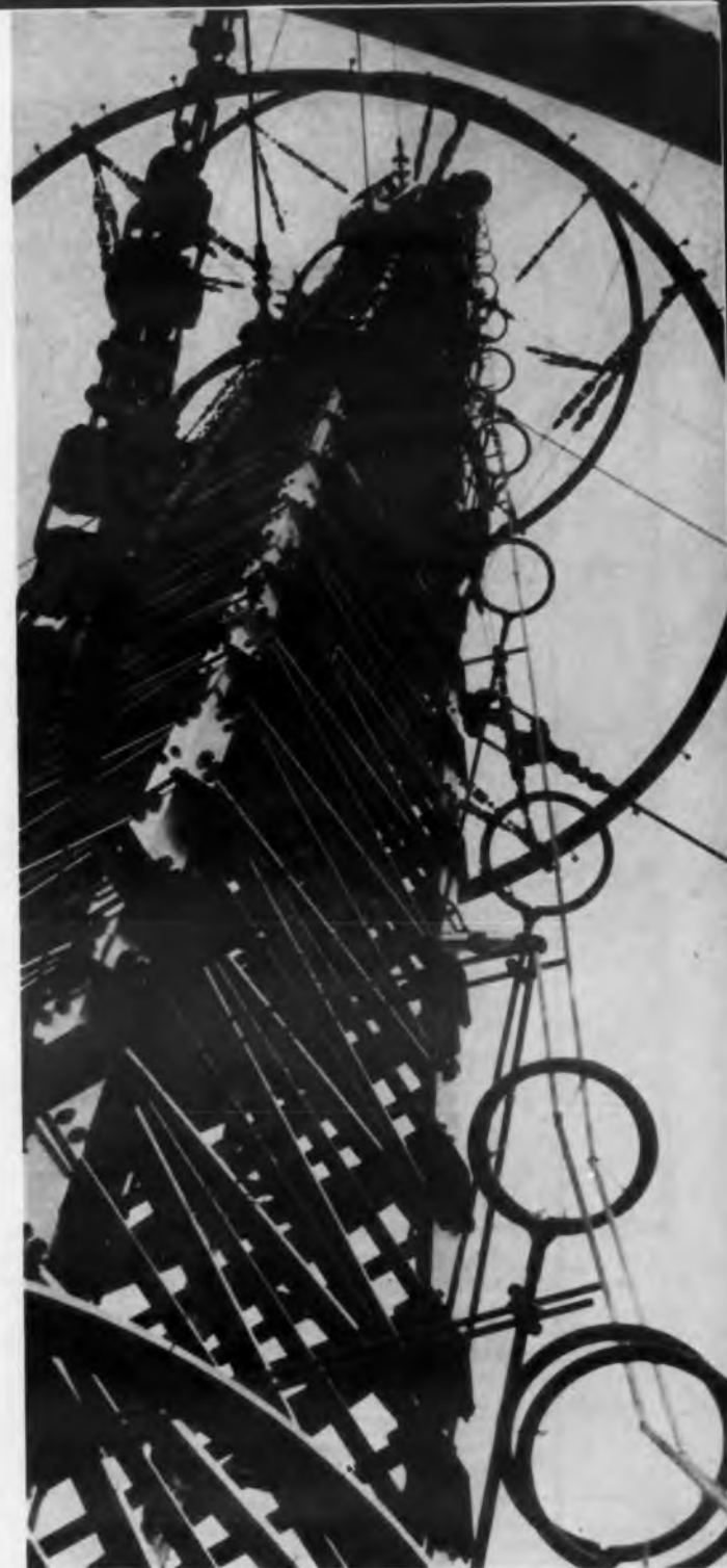
Surface-wave antenna line on German television transmitter. The G-line is supported within the metal rings by nylon cords. Note the parallel coupling method used (lower half of photo) between two G-lines in close proximity. Such applications, while popular abroad, have lagged in this country despite major cost savings claimed for the G-line. Renewed interest in uhf television may, however, provide new impetus for G-line use here.
