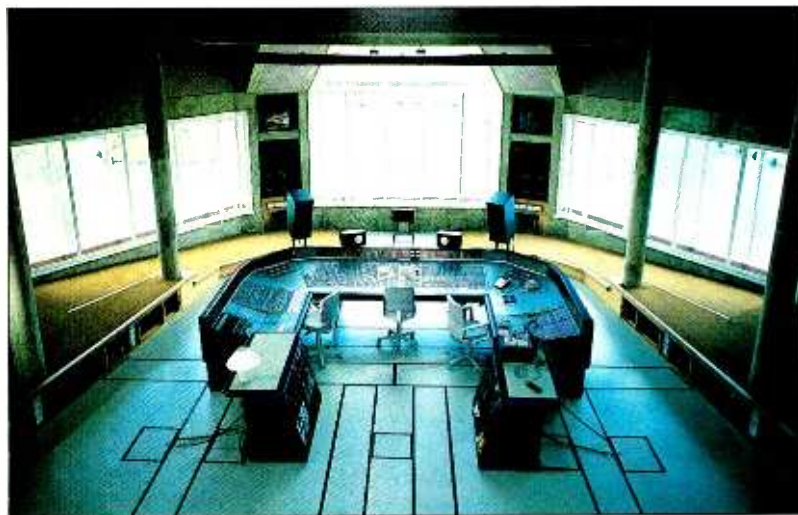
Control Room One
