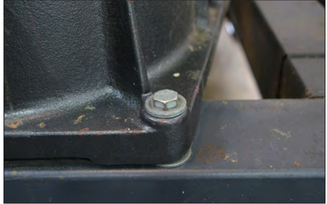
3 - A washer was inserted between the lathe and the stand to fill the gap, before tightening the mounting bolt.
