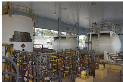
Pictured Left: Seismic Improvements with Chemical Hypochlorite system at the Harry Tracy WTP
