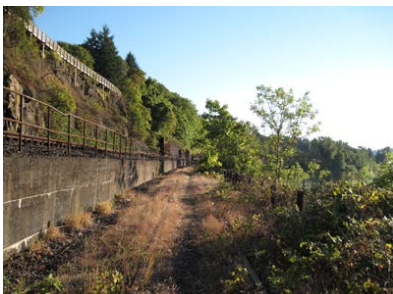
Rail spur adjacent to the Union Pacific railroad and Hwy 99E above
