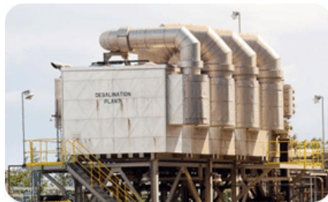
Tampa Bay, Florida, has one of the few desalination plants in the United States.
