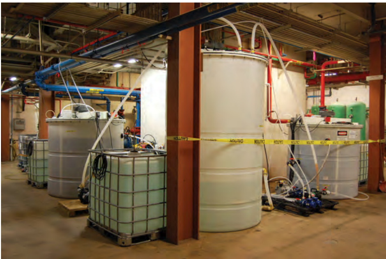
The pilot-scale demonstration of the CANDO process for converting ammonia to nitrous oxide for energy recovery.
