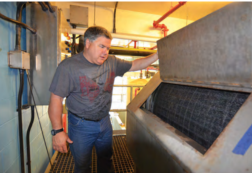
Dave Garabedian, operations and maintenance specialist, checks the shear mixer after the chemical bond between the floc and magnetite has been broken.
