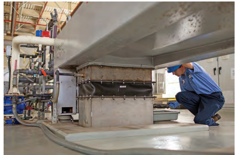
Michael Bonifacini samples biosolids from the plant's heat dryer.
