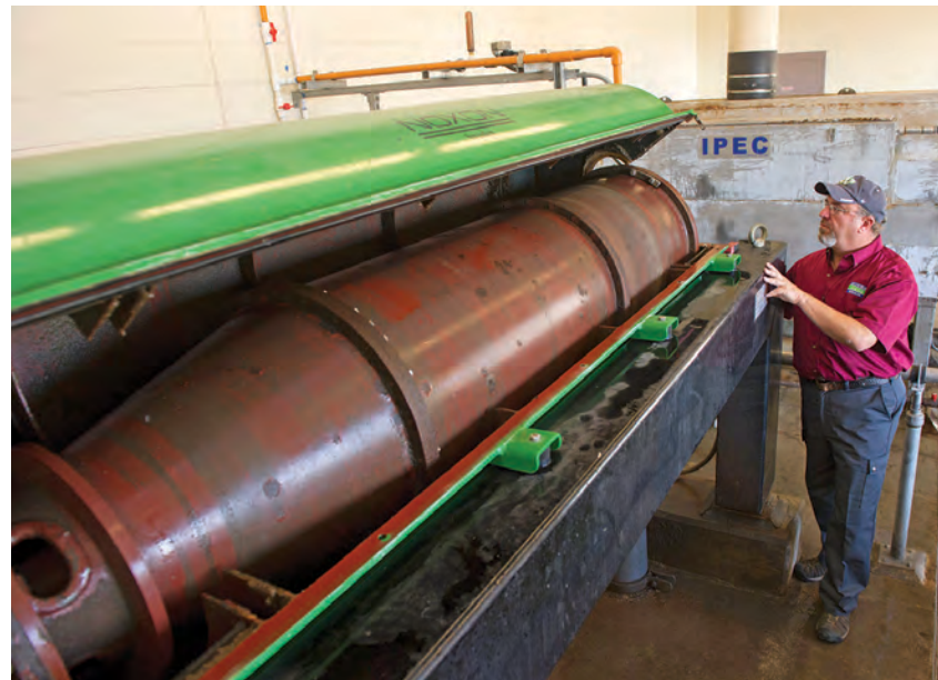
Thickened sludge from the plant's digester is pumped to a high-speed decanting centrifuge from Noxon (shown) for dewatering. Polymer aids in liquid/solid separation.
