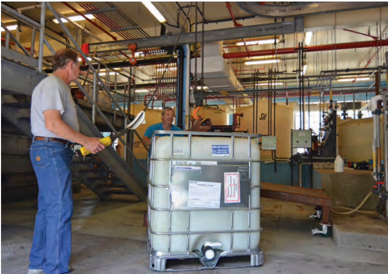
Operators Jim Lucas (left) and Ken Richard position a container of Kemira Superfloc polymer for dewatering biosolids.
