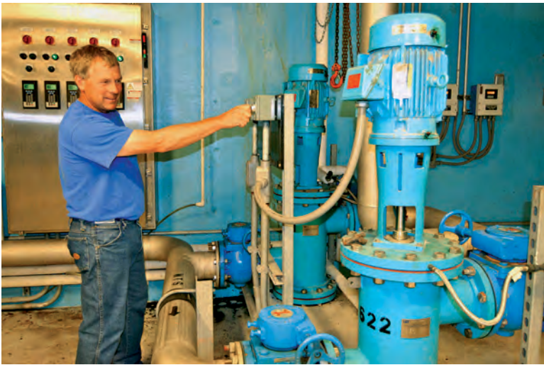
Jeff Kalmes, plant supervisor, swaps out the shear mixers that separate magnetite from floc before the CoMag influent enters the magnetic recovery drum.
