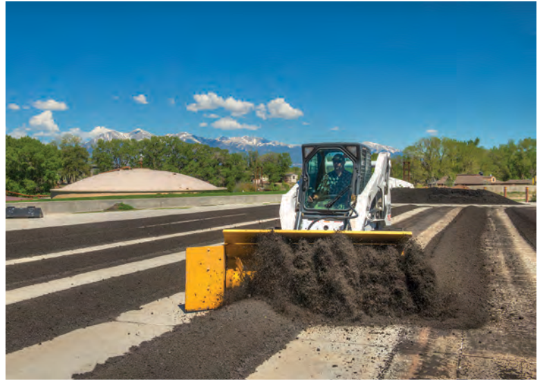
ABOVE: Windrowed compost piles are turned as necessary. LEFT: Deep in the Rocky Mountains, the Salida Wastewater Treatment Facility received the 2013 Plant of the Year Award from the Colorado Rural Water Association.
