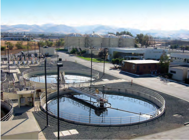
Secondary clarifiers at Delta Diablo, which serves 42 square miles with a population of 200,000 in Antioch, Bay Point, and Pittsburg. The sanitation district was formed in 1976, and the plant went online in 1980.
