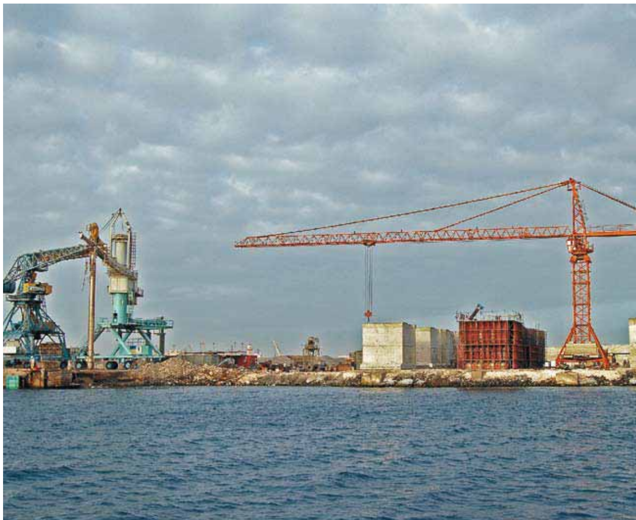
A major extension to the Port Sudan harbour, known as the Green Port, is going ahead in an area surrounded by seagrass beds and coral reefs. It is now necessary to focus on planning port operations to minimize ongoing impacts
