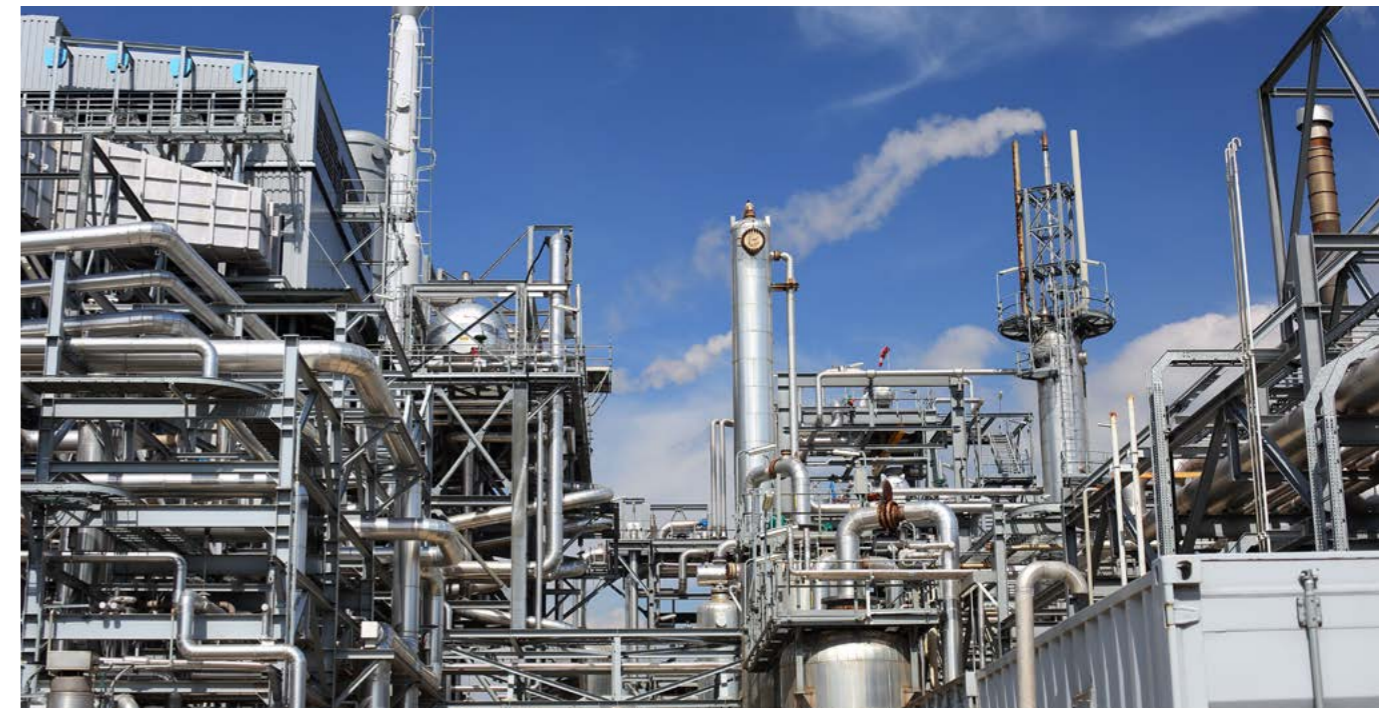
Hydrogen plant in The Netherlands depicting Technip Energies' technical capabilities in the refining industry.
