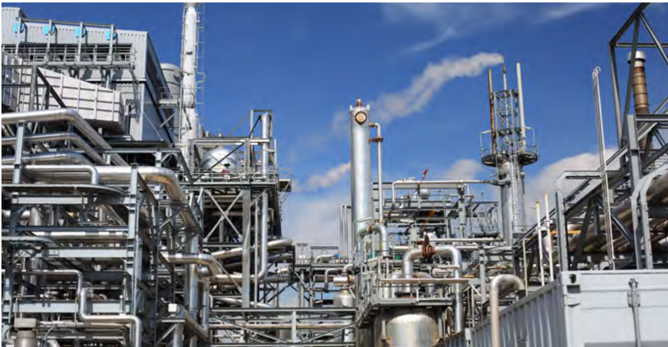
Hydrogen plant in The Netherlands depicting Technip Energies' technical capabilities in the refining industry.
