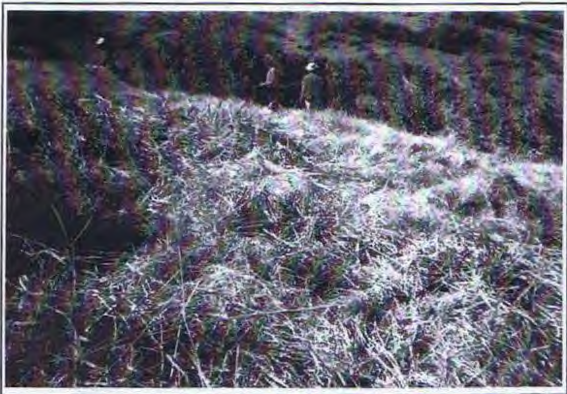
PHOTOGRAPH NO. 19 N.W. Peninsula. NP-23, From East Side of Grid After Grubbing.
