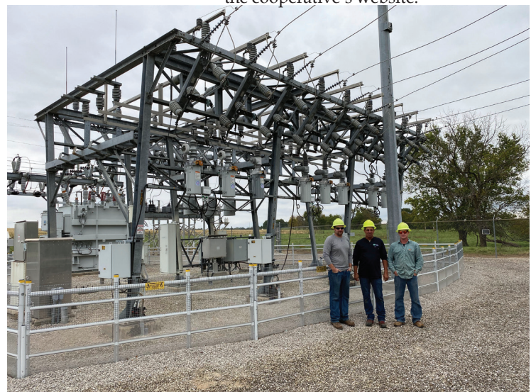
Jared Asmus, Randy Fletcher, and Josh Heiserman after completing work on reclosers in the El Dorado Springs substation.
