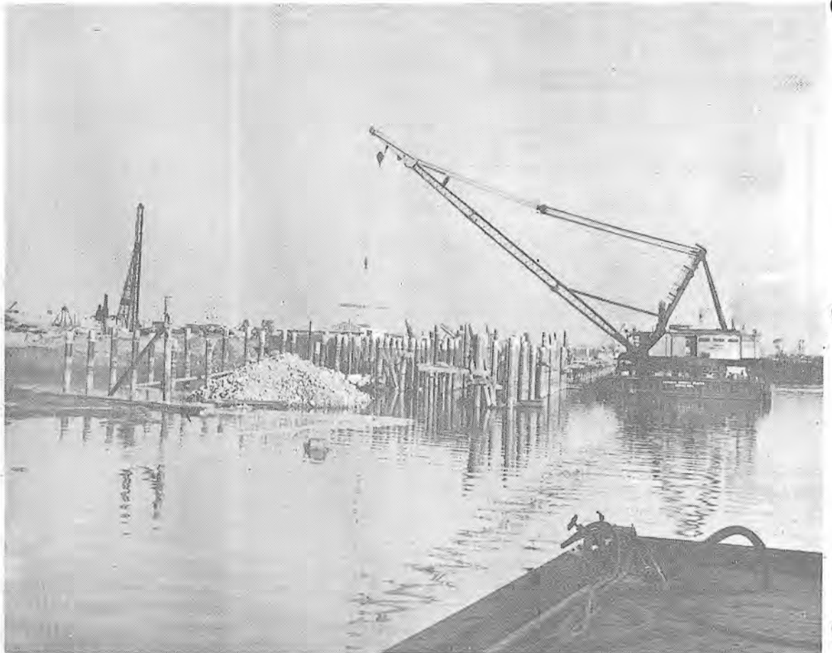
HARBOR IMPROVEMENT —new harbor facilities at the foot of Marina St. in San Francisco are being installed by Manson General Co. This floating barge has been on the job around the clock for several months. In foreground is seen the several hundreds of concrete piles while pile driving is at left background.
