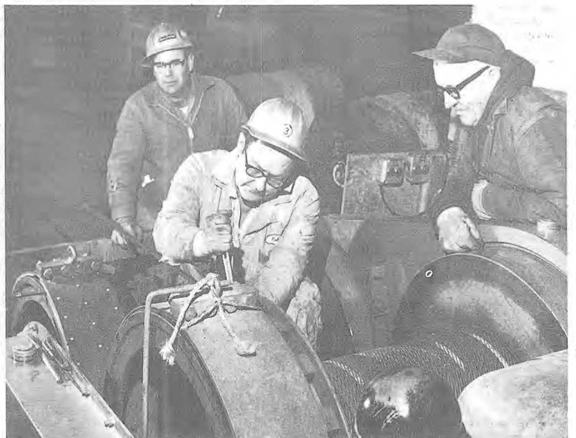
TIME OUT —this crew at Wells-Fargo bank building handles two-drum hoist at the 44th-floor structure being built. Here is an example of how brake drum is kept clean by use of manila line tied to rig.
