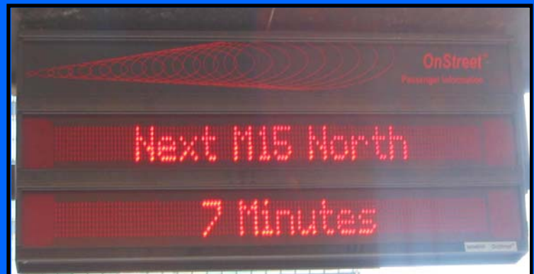
Newly Installed Passenger Information Sign at Bus Shelter in Manhattan
