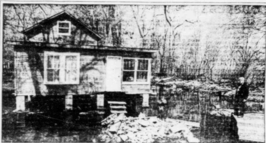
Put-In-Bay Mayor Steve Urge checks an island cottage that had to be raised and moved sideways to save it from the ravages of high Lake Erie waves. PHOTO BY RICHARD ELLIOTT
