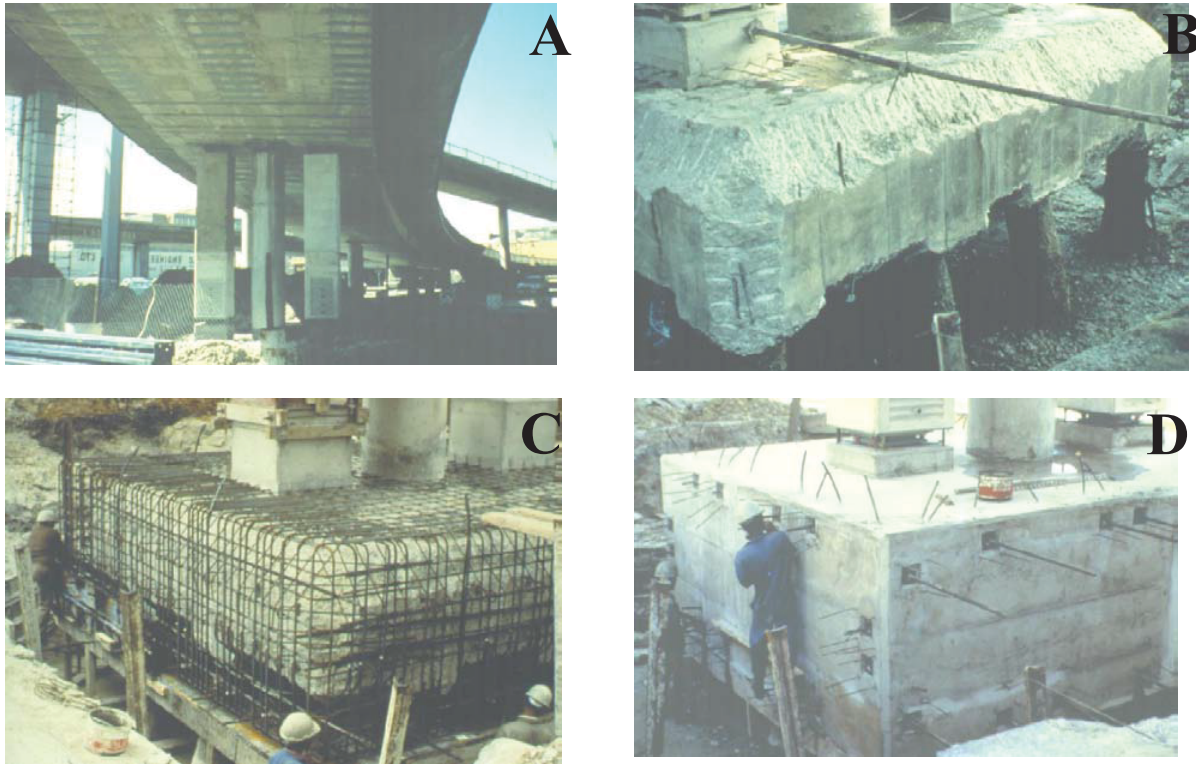
Figure 8. (A) Series of photographs showing strengthening of ASR-affected bridge in South Africa (after Fournier et al. 2004). (B) General view of a highway structure affected by ASR in South Africa. Cracking due to ASR was observed in the pile caps supporting reinforced concrete columns. The cracked concrete was first removed. (C) Additional steel reinforcement was added around the pile cap. (D) External strengthening was provided by means of prestressed cables. (Photos courtesy of R.E. Oberholster, PPC Technical Services, Cleveland, South Africa)
