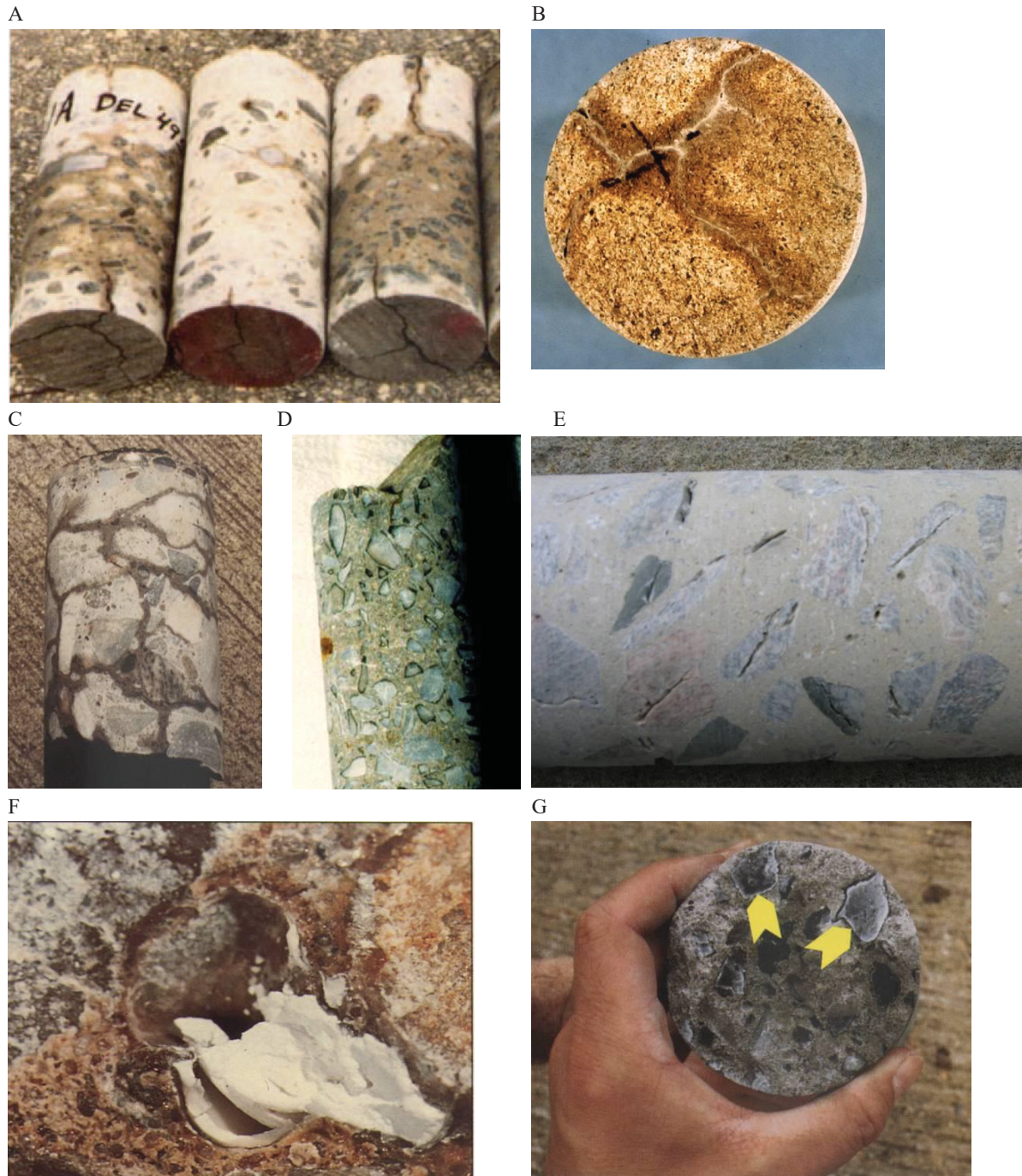
Figure C1. (A). Cores extracted from a concrete pavement affected by ASR and showing macrocracks penetrating from the upper and lower parts of the pavement. (B). Gel staining surrounding cracks and gel exudations at the surface of a core extracted from a sidewalk section affected by ASR (C). Fine cracking pattern showing up after re-wetting of the core. (D). Dark rim around the periphery of reactive aggregate particles. (E). Macrocracks in reactive coarse aggregate particles. (F). Deposits of alkali-silica gel in a void on core surface. (G). Deposits of alkali-silica gel on the broken surface of a core extracted from a highway bridge structures affected by ASR.
