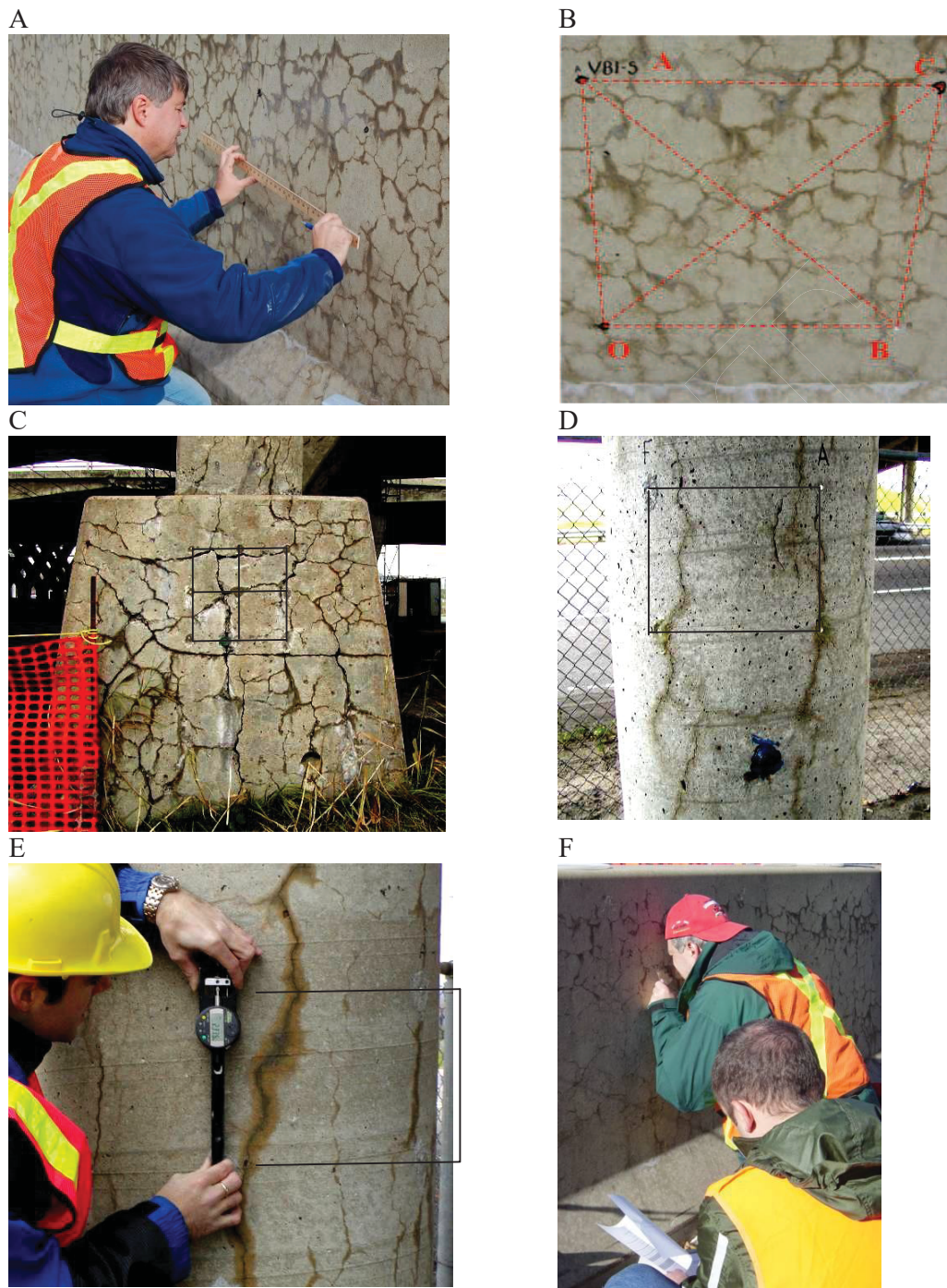
Figure B2. (A and B). Laying out of the reference grid on a concrete median barrier affected by ASR. (C). Four small reference grids are drawn on the exposed surface of the foundation block of reinforced concrete columns of a highway bridge structure affected by ASR. (D). Reference grid on the exposed surface of a reinforced concrete column of a highway bridge structure affected by ASR. (E). Expansion measurement at the surface of the above concrete column. (F). Cracking Index measurements.
