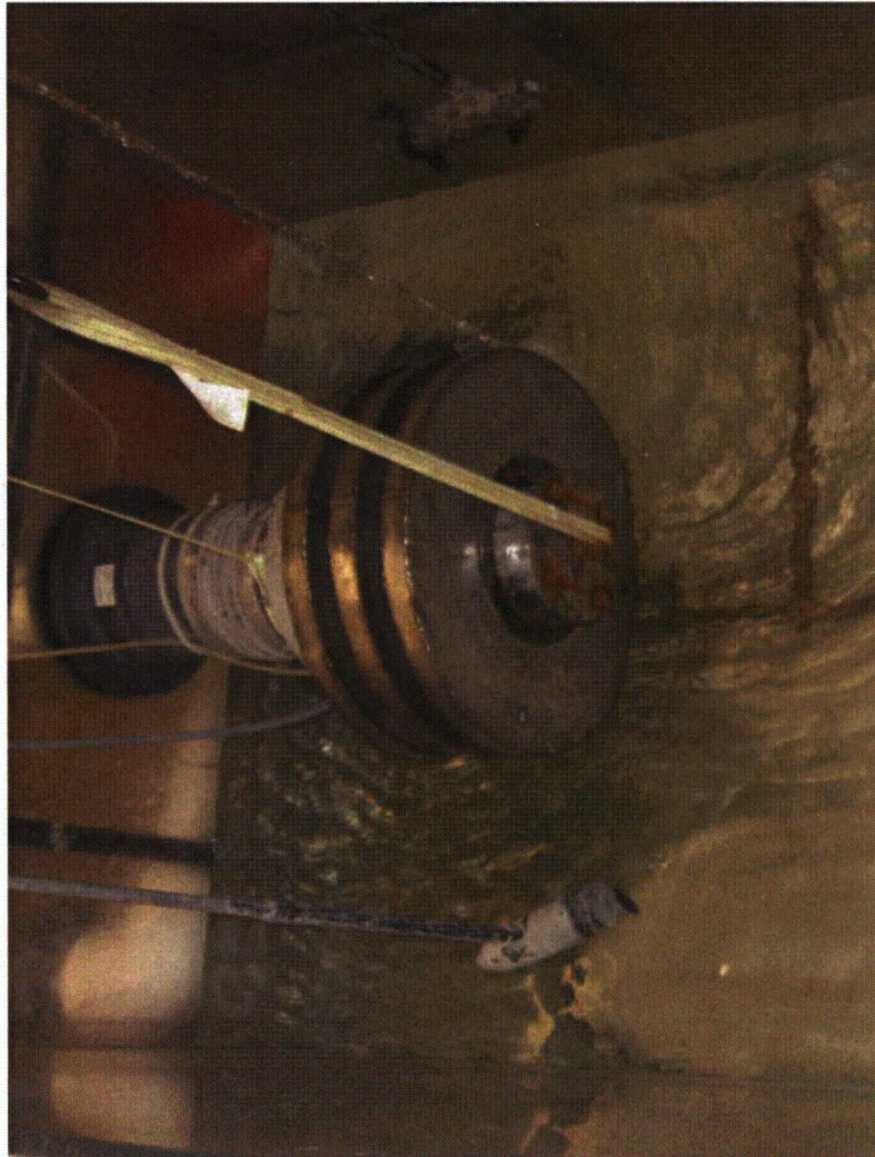
Figure 4-8 – Photograph of PCI Strainer with Mechanical Mixers
