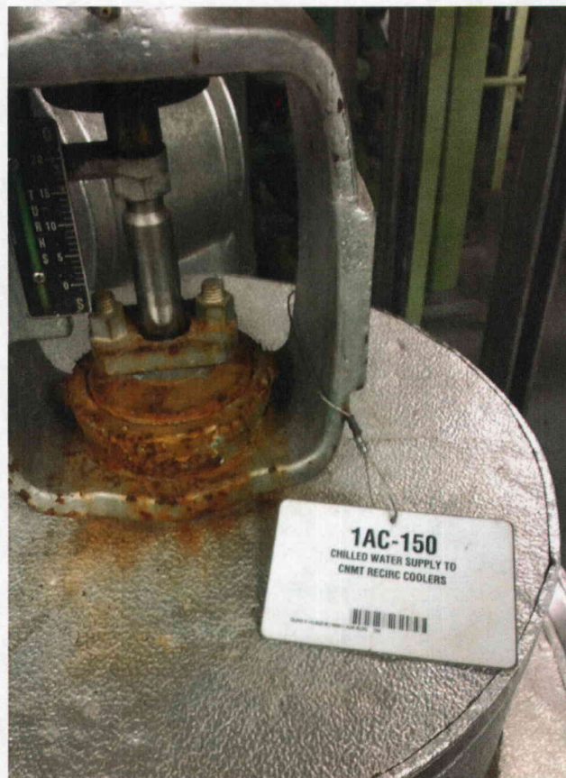
Figure 6-1: Surface corrosion for valve 1AC-150
