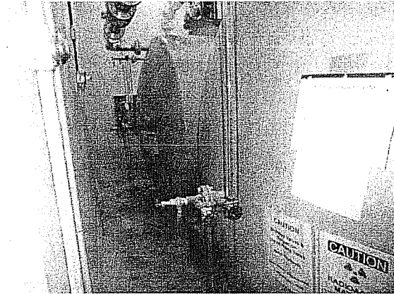
Figure 5, Two Waste Tanks in Room B045
