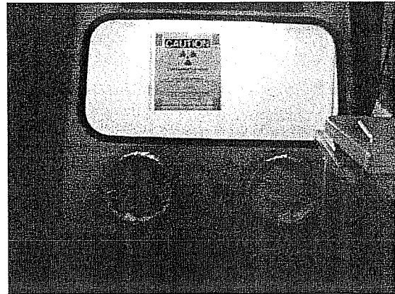
Figure 22, Contaminated Glove Box in PU Area
