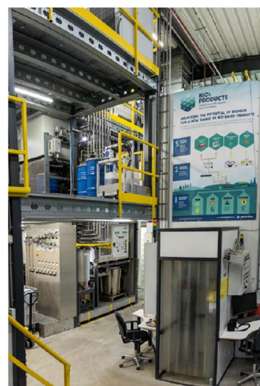
Figure 14: BTG's 3 tonne/day pyrolysis oil fractionation demo plant
