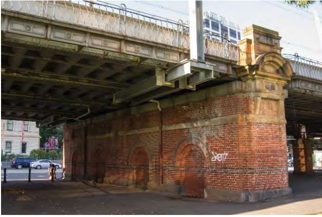
Figure 14. Brick structure with decorative sandstone end pediment (corner Market St). (Source: Context 2019)
