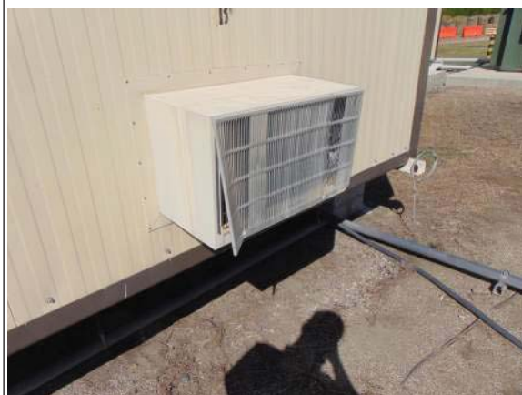
Photo #57: Typical Deficiency: air conditioner fins bent and obstructed
