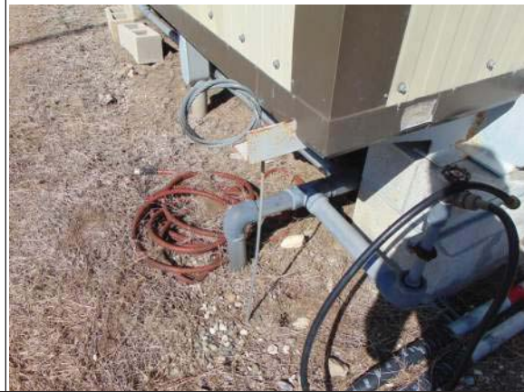
Photo #68: Typical grounding arrangement: 6 per CHU
