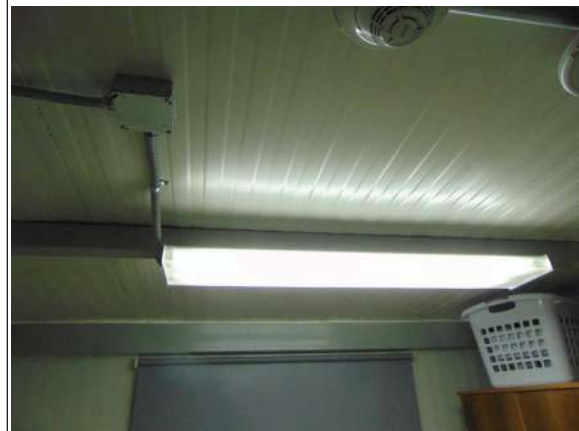
Photo #64: Typical overhead fixture - Bedroom
