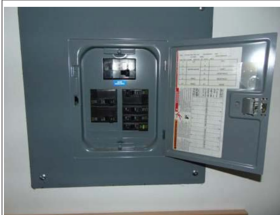
Photo #61: Typical electrical panel (100A Service)
