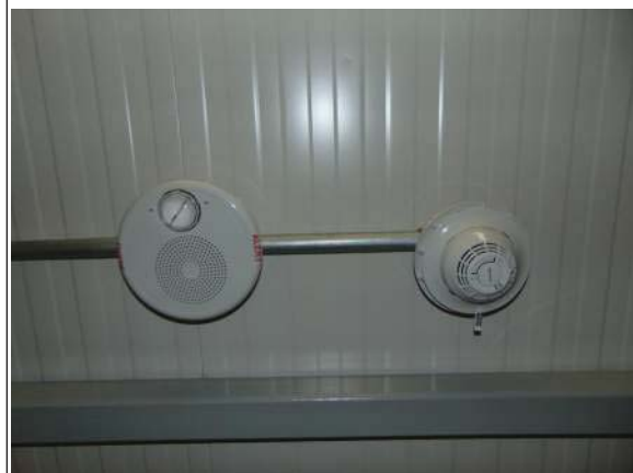
Photo #72: Typical Interior fire detection/alert system
