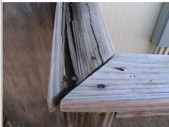
Photo #29: Replace all pressure treated wood railings
