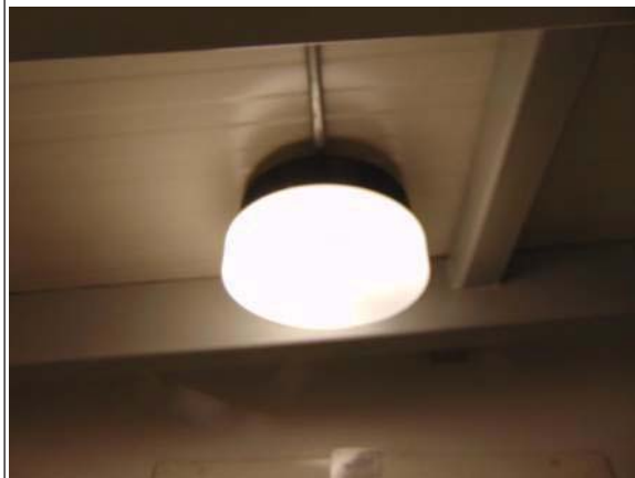
Photo #65: Typical overhead fixture - bathroom
