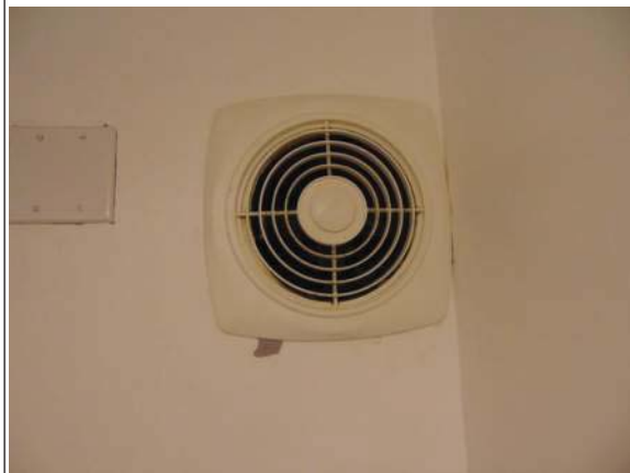
Photo #69: Typical Exhaust Fan (See Photo 66 for hood)
