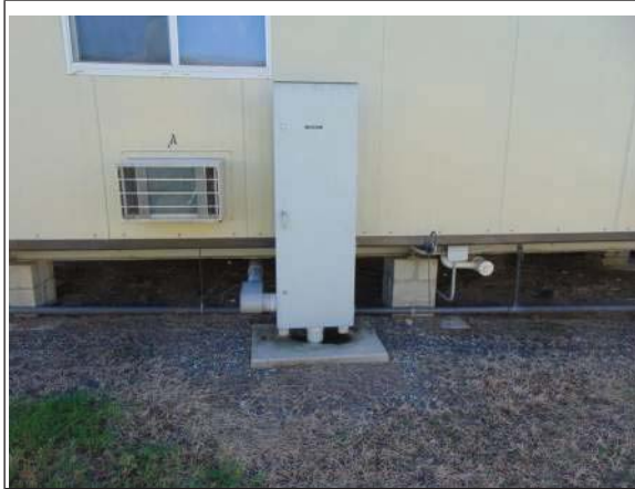
Photo #67: Typical electrical distribution: 1 panel per 6 CHU's
