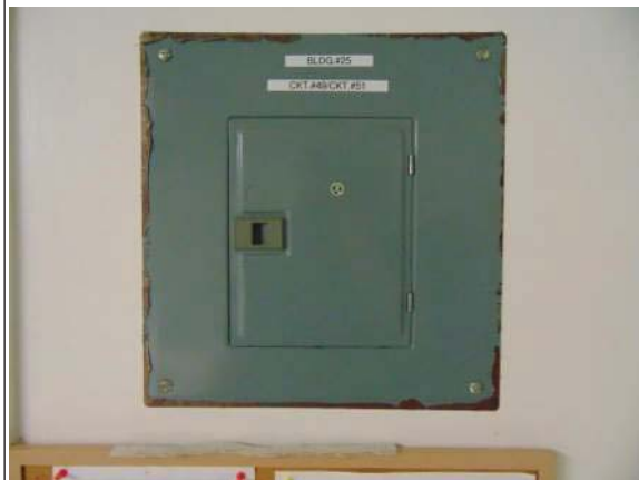
Photo #63: Typical electrical panel - closed
