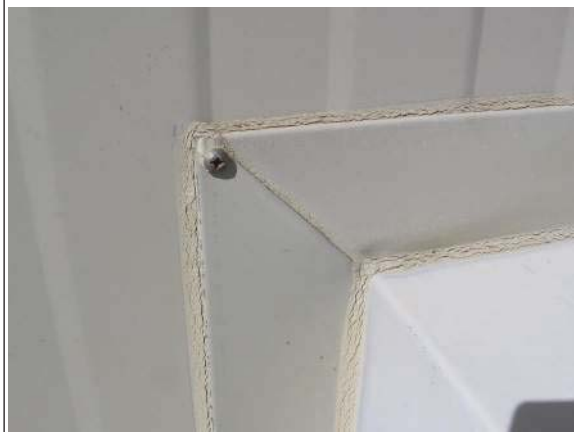
Photo #17: All exterior penetrations need to be re-caulked
