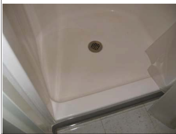
Photo #13: Typical fiberglass stand-up shower fixture
