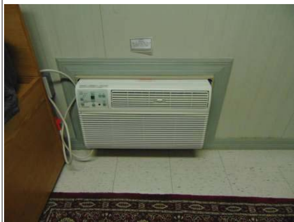
Photo #59: Typical Air Conditioning Unit
