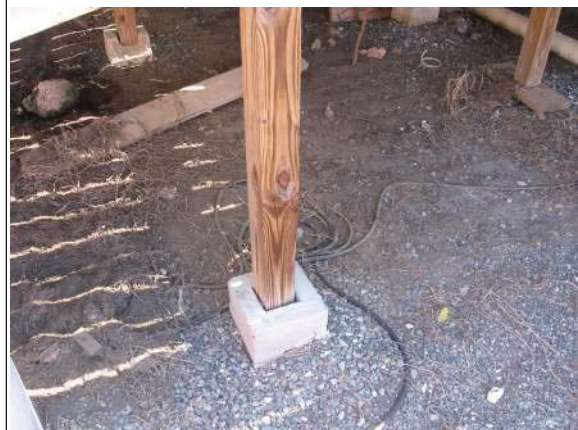
Photo #30: Typical pressure treated wood post on concrete piers supporting deck structure
