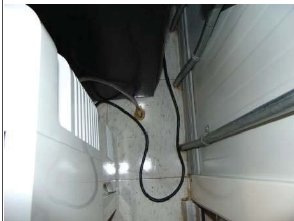
Photo #71: Typical dehumidifier drain-line floor penetration
