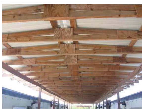
Photo #25: Typical exterior covered pressure treated wood truss and metal roof system
