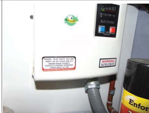
Photo #56: Water-heater name plate
