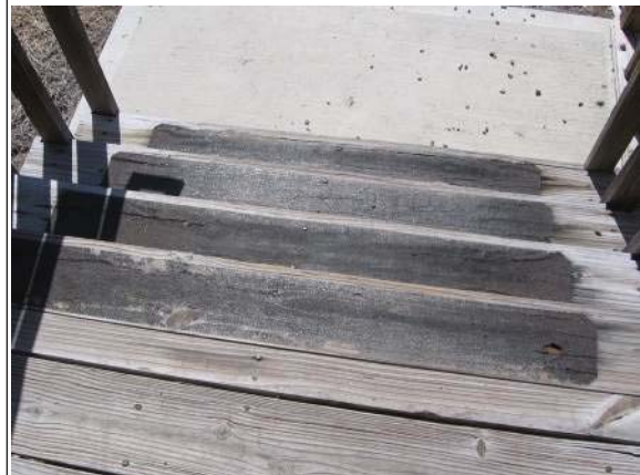
Photo #28: Replace all slip resistant stair tape
