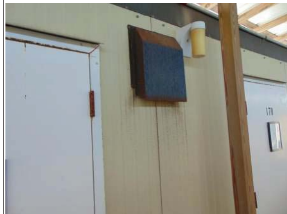
Photo #66: Typical exterior fixture
