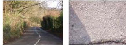
Broken Concrete (vehicle speed 50 Km/h)
