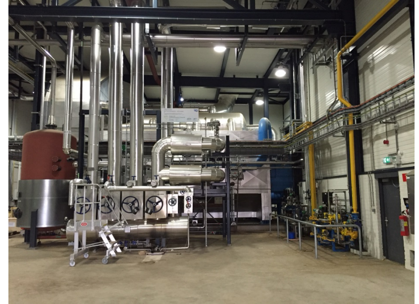
FPBO boiler at FrieslandCampina
