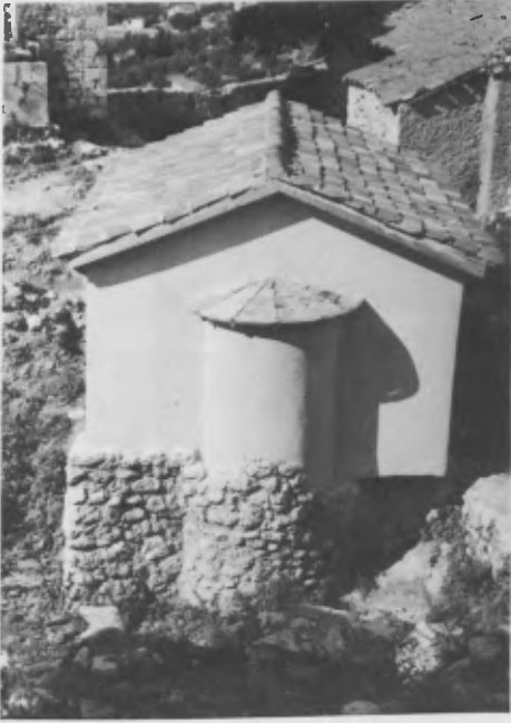
Figure 5. The SW side of the castle: definitive conservation of the 9th century chapel, re-creating spatial volume.
