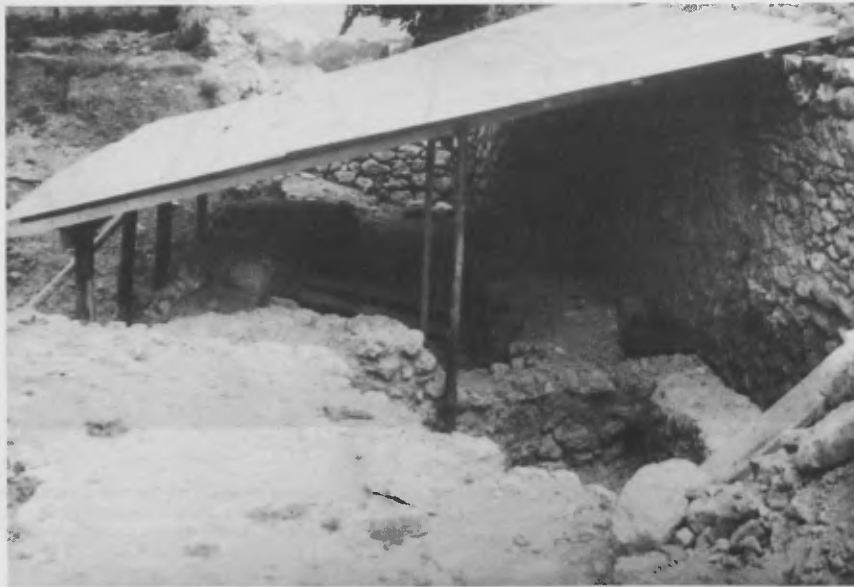
Figure 4. The SW side of the castle: the 9th century chapel. Temporary protection during excavation of painted wall plaster was provided by a very simple shed with corrugated asbestos cement.
