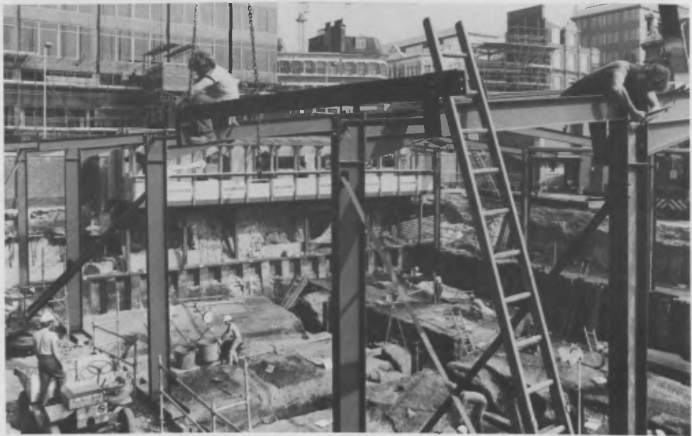
Figure 3. Billingsgate, City of London, 1982: as winter approaches, a temporary roof is built over the excavated area. It has open sides and ends to allow cranes to remove the spoil from the excavation (Museum of London).
