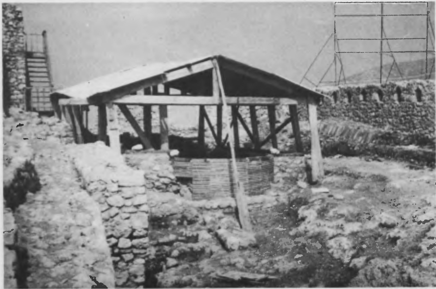
Figure 12. Acropolis: temporary roof before starting excavation in the interior of the churches near the donjon.
