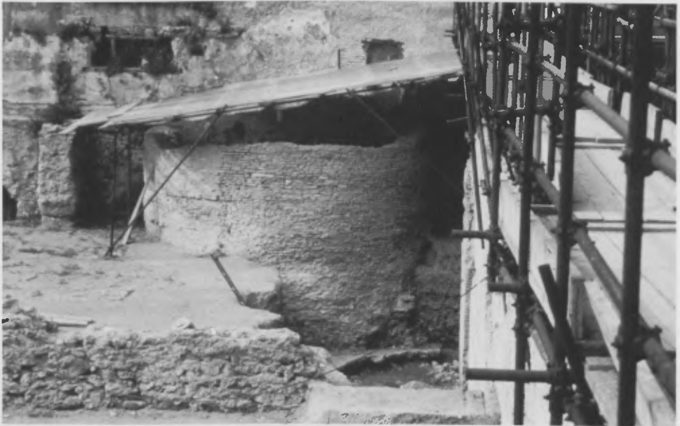
Figure 2. Wall of mudbrick laid in clay. General view showing the temporary shelter of metal tubing, corrugated plastic and bamboo screening. This roof serves to keep off rainwater and to limit insolation, overheating and drying of the clay. The wall is about 4 m high. Photo: author.
