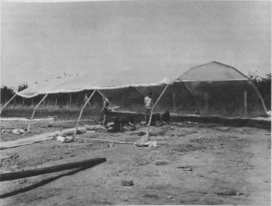
Figure 2. Work in progress under shelter with front edge of polyethylene sheet rolled up during fine weather.
