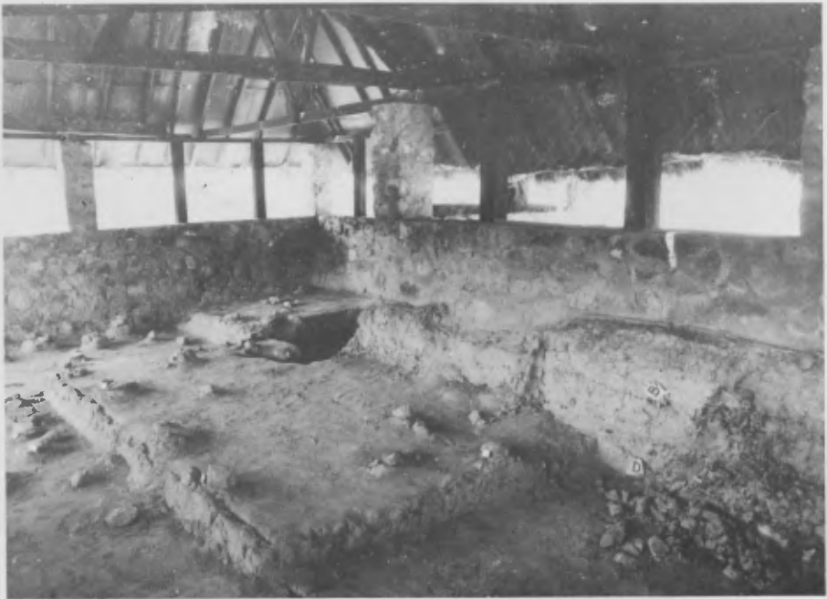
Figure 8. Artifacts displayed in situ in on-the-spot museum; note decay of wall base.
