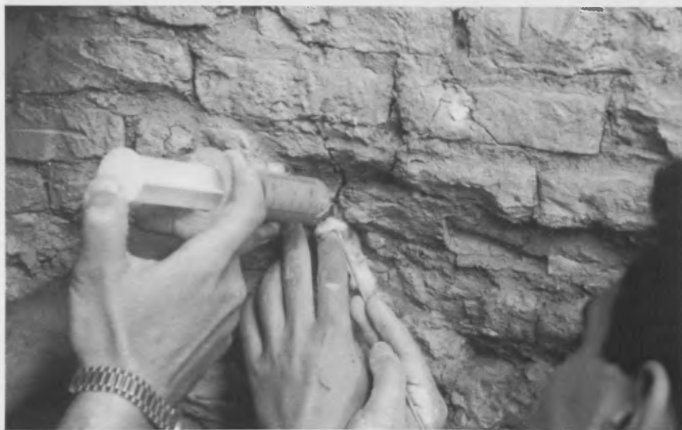
Figure 6. Consolidation with infiltrations of a clay solution combined with 10% hydraulic lime. Photo: author.
