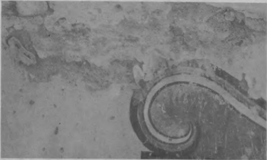
Figure 4: Painted plaster in Sanctuary. Note the paper along the top edge of the painted volute that was used in an attempt to temporarily reattach the paint film to the plaster ground. NPS photograph, 1976.
