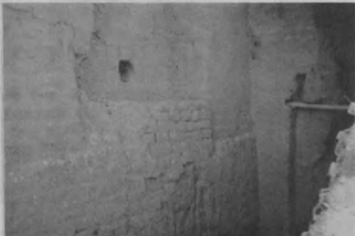
Illustrating problems of decay Surface spalling on an interior wall.
