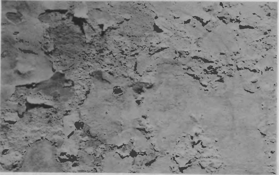
Figure 5: Plaster surface with extensive deterioration by efflorescence forming on the surface and immediately beneath the paint film. NPS photograph, 1979.
