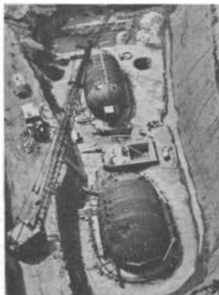
Installation of underground control center for Minuteman missile launching facilities at Grand Forks Air Force Base, North Dakota.
