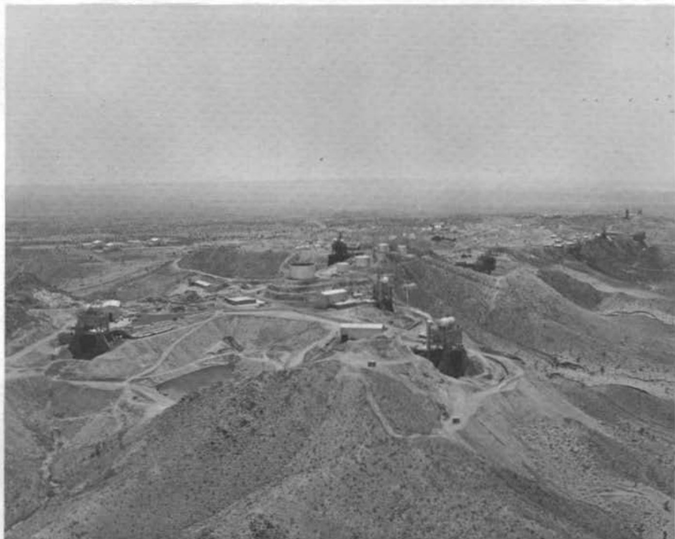
Photo shows new three F-1 test stand addition at NASA High Thrust Area, Edwards California, constructed under supervision of the Los Angeles District, U. S. Army Corps of Engineers. Test Stand 1-E is on left with water recovery reservoir. Also shown is Test Stand 1-D in foreground right and Test Stand 1-C adjacent.
