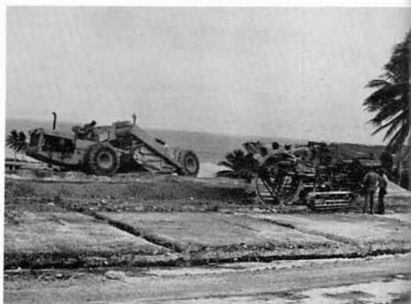
Fine grading, ditching, and much more was required before the concrete was poured.
