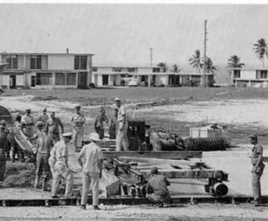
The TM's dump their load, and the concrete men and screeder go into operation.
