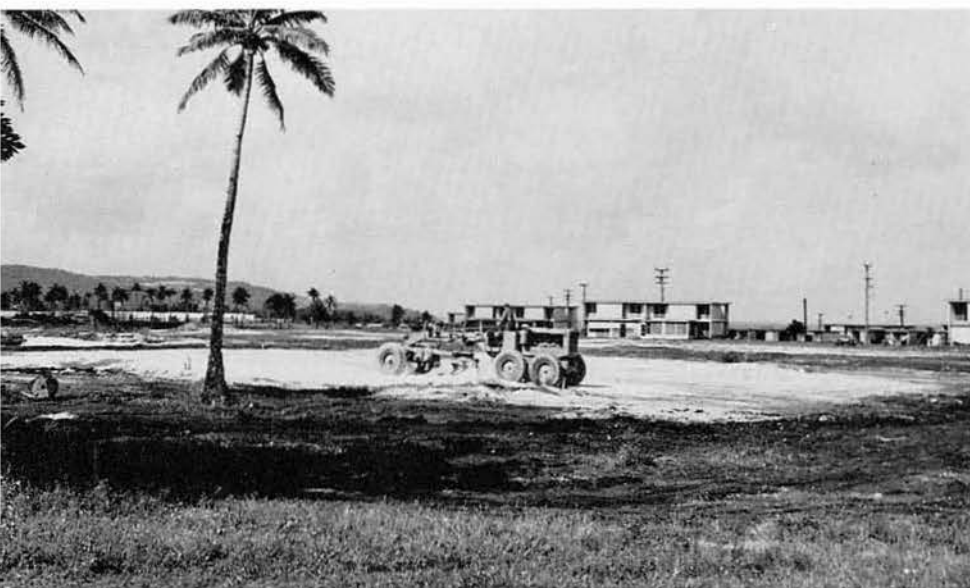
We were given a few patches of land and told to build a bunch of houses, so let's get started.
