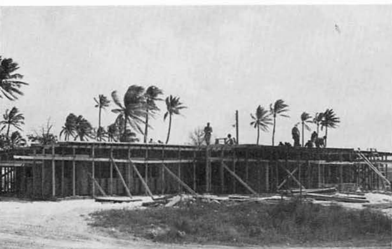
The crew finishes off the roof form in preparation for re-bar work.
