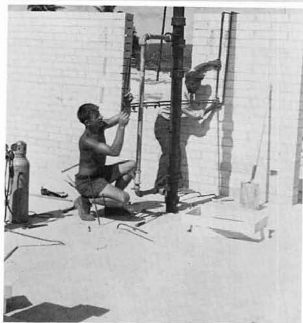
and up goes a vent pipe with the rest of the plumbing.
