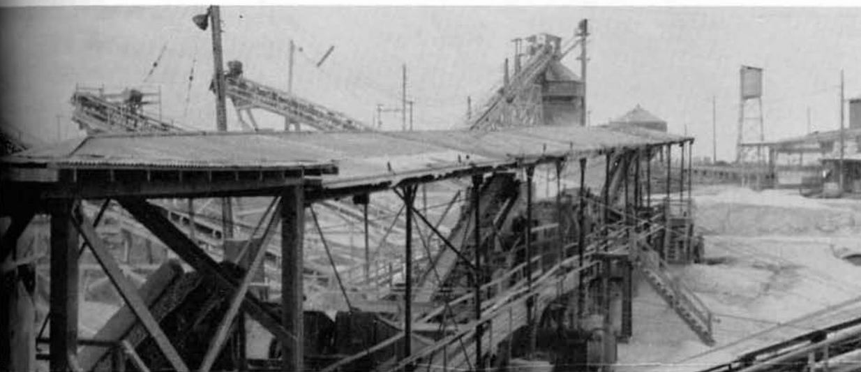
The "A" Crusher. October '58, and Eleven's Bees moved in with parts, new ideas, ambition, and a little cussing. The end result—a dead skeleton becomes a live monster and the crushed coral starts piling up.
