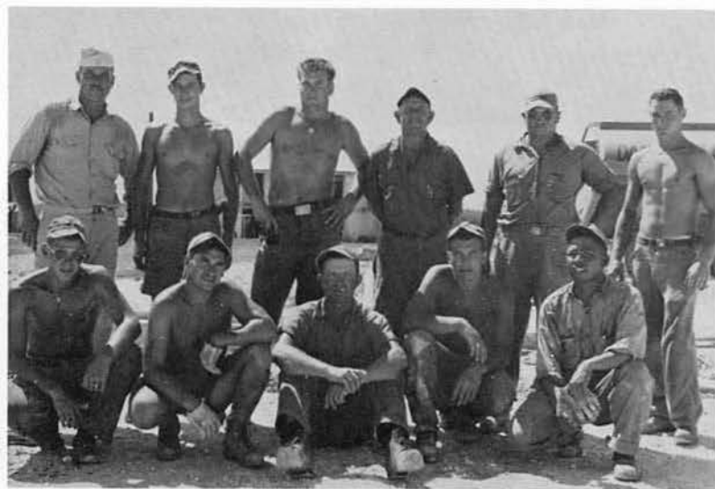
The Re-bar Crew. The men who laid and tied re-bar for over a hundred concrete pads.
