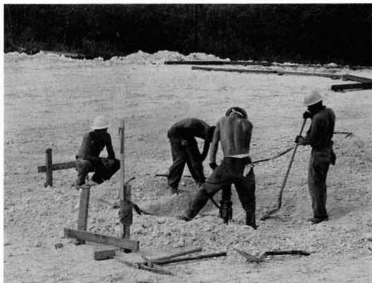
The Butler Building's coral pad is finished and the jack-hammers move in to knock out foundation space.
