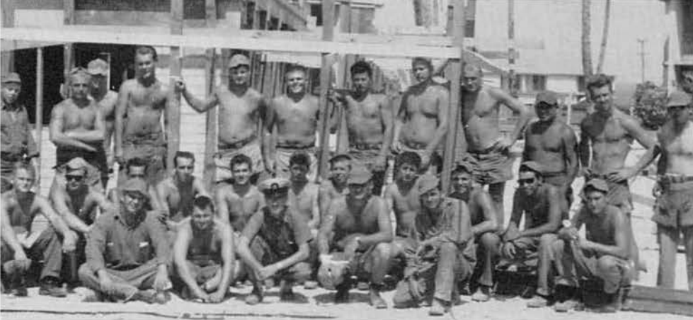
Roof Form and Re-bar Crew. All they asked was for enough lumber, then the rest was a breeze for them.
