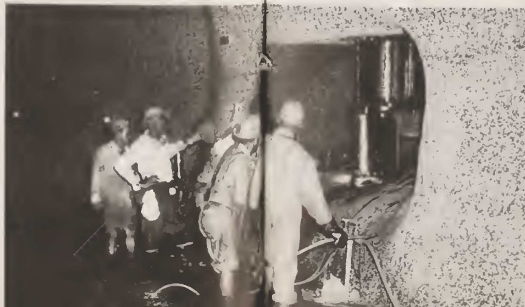
A group of employees in the center culvert of one of the cylindrical valves. There are 40 of these valves opening off the Miraflores Locks centerwall culvert, none in the east or west lanes culverts, where rising stem valves provide water control necessary. Gatun Locks have 60 cylindrical valves, and Pedro Miguel Locks, 20.
