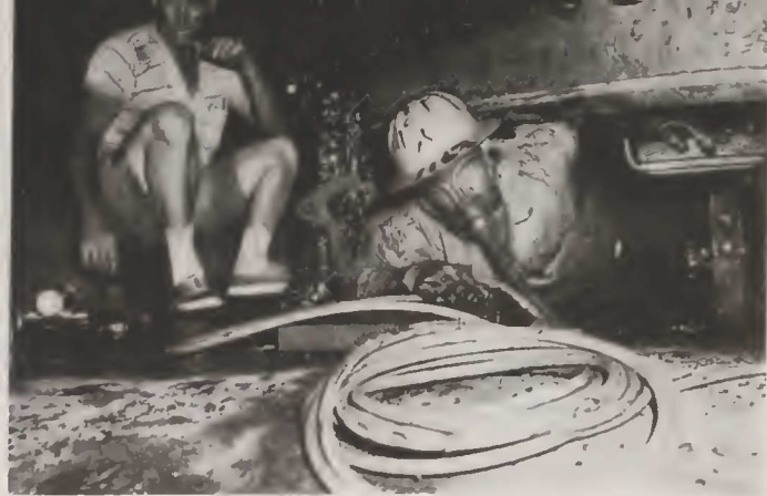
Wearing a mask with air hose line attached, Armando González crawls out from under one of the huge cylindrical valves. Masks with air hose attachments are worn by workers in restricted areas where fumes effects might result. Visible on the left support of the valve is one of the heavy steel brackets which assure that the valve's inside "drum" remains elevated while work is in progress. At left is McNair C. Lane, lead foreman painter.
