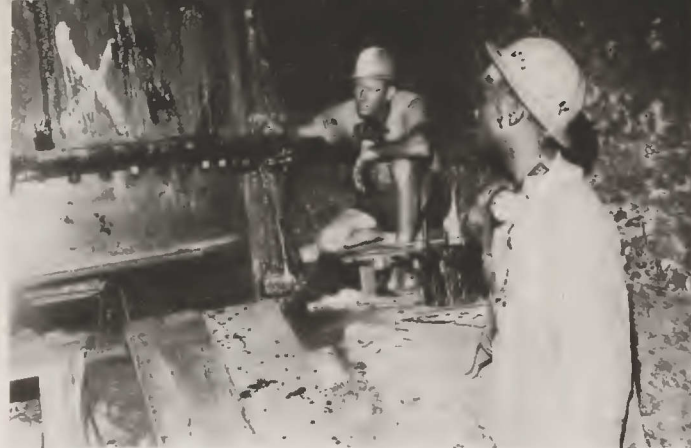
Robert E. Budreau, lead foreman painter, checks cleaning and painting work on one of the cylindrical valves. Visible just below his right hand are the large nuts holding in place the iron segments which retain the rubber seals which bear against the inner moving "drum" section of the cylindrical valve. At right is George W. Pinnock.
