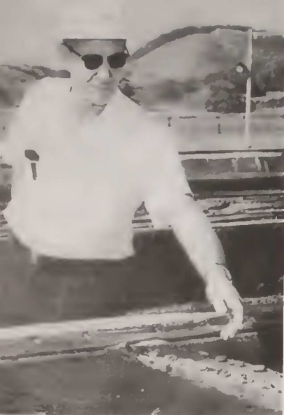
Truman H. Hoenke, in charge of the Miraflores Locks overhaul, points to rivet head corrosion on one of the old style riveted rising stem valves taken from the centerwall culvert. Eighteen all-welded valves are being installed during the current overhaul, completing a changeover to this type started during the 1958 overhaul. Mr. Hoenke is Locks Superintendent, Pacific Branch. This is the 6th locks overhaul in which he has been involved.
