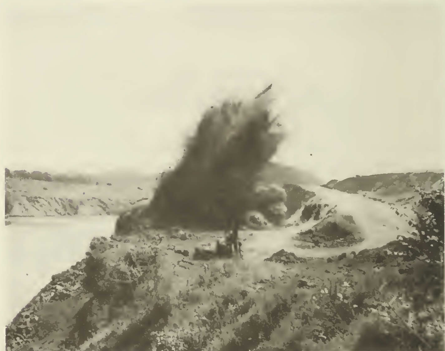
The blast of the rock wall. Note how the planned loading and detonation has caused the rock to be thrown away from the Canal waters and back into the quarry pit, and the safe location of the contractors' equipment and absence of any craft in the Canal.
