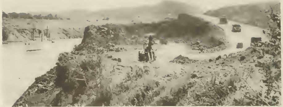
A high, badly fragmented "fly rock" wall standing almost vertically above the Canal waters. This must be broken (blasted) in such a way as to minimize the amount of fractured material which falls or is thrown into the Canal. Also shown are a passing ship and the contractors' equipment. These must be carefully considered before detonation of a blast.
