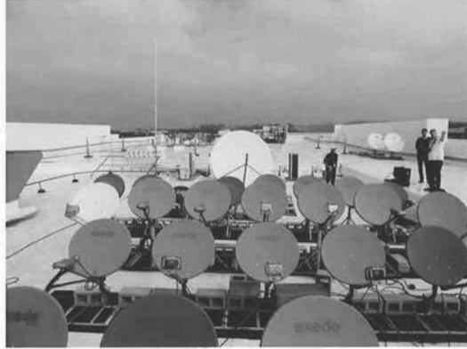
View of transmit antenna looking north
