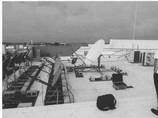
View of transmit antenna looking west
