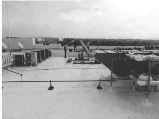
View of transmit antenna looking south
