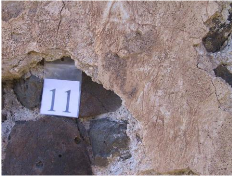
Fig. 19 - FOG-M11 sample – external finish coating
