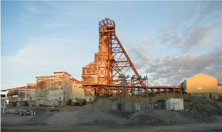
Figure 2: Giant Mine Shaft no. 2 headframe partially deconstructed, July 2012. The mine site is currently undergoing extensive subsurface and surface remediation. Photo by Kevin O'Reilly.
