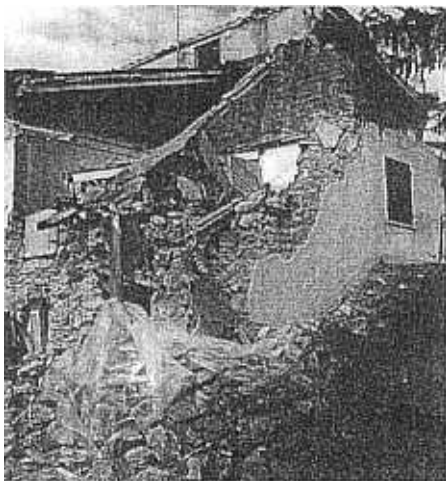
Figure 12 - Typical damage to vernacular architecture in Umbria-Marche, Italy. (photo: Tobriner)
