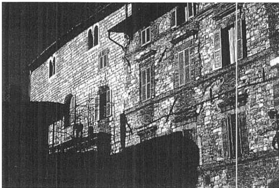
Figure 5 - Exterior anchors and tie bars on masonry buildings are a distinctive feature of Assisi vernacular architecture. These early mitigation efforts demonstrated their effectiveness in this quake. In this photo, the wall on the right, with anchors and tie bars, is intact and plumb, while the un-anchored wall on the left is cracked and bowing outward.
