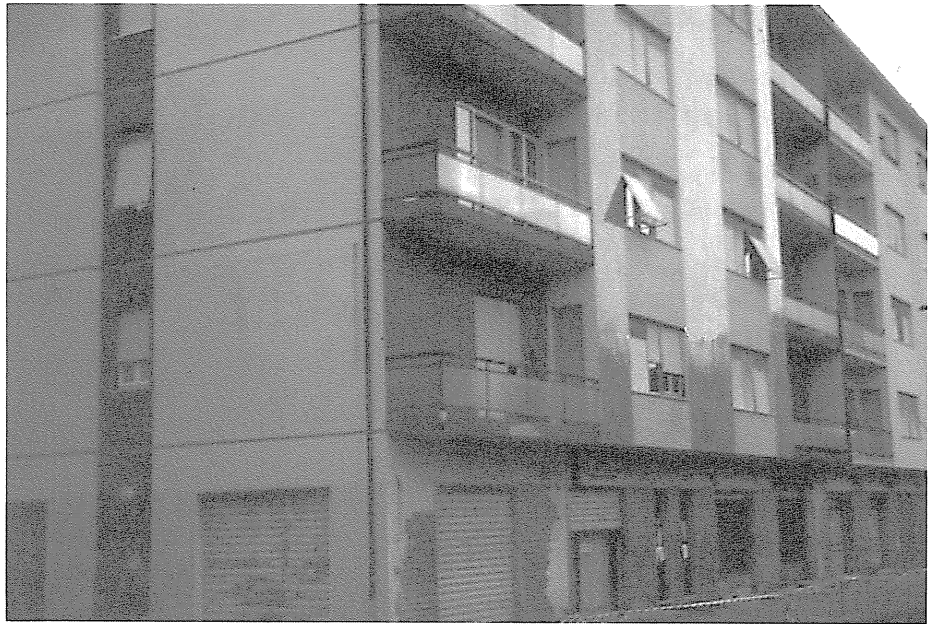
Figure 6 - These modern concrete apartment buildings had been vacated. Exterior damage consisted of spalled and cracked concrete. (photo: Tobriner)
