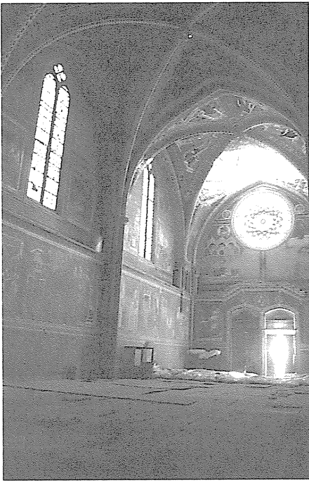
Figure 10 - The interior of S. Francesco in Assisi, showing the collapsed first vault (above the rosette window). (photo: Tobriner)
