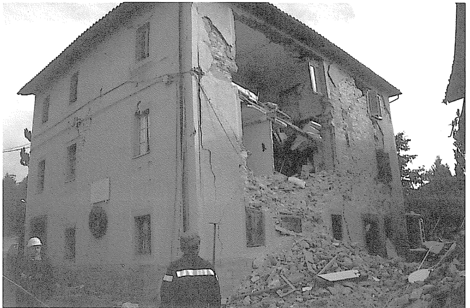
Figure 7 - This building in Cesi illustrates typical damage suffered by the area's vernacular architecture: exterior wall failures in stone masonry buildings. (photo: Tobriner)
