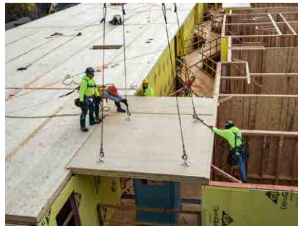
Figure 7. The Canyons CLT and light frame integration. Source: (Marcus Kauffman, Oregon Dept. of Forestry n.d.)
