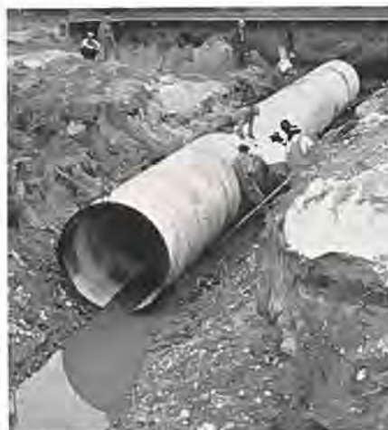
Showing installation of 72-inch corrugated culvert under three railroad tracks near Fort Collins.
