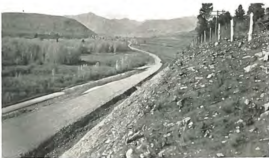
Another big improvement was made on the road between Durango and Mancos in 1931 with the completion of the project, at Hesperus as shown by above view. Photo by U. S. Bureau of Public Roads.
