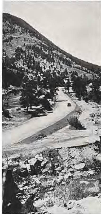
View of new Ute Pass highway near Cascade with old road at the right. Photo by V. H. Littlefield.
