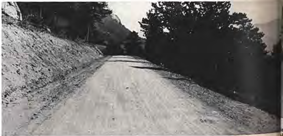
Showing a section of the new road being constructed by the Forest Service over Willow Creek Pass, leading into the North Park country from the Colorado River, near Granby.
