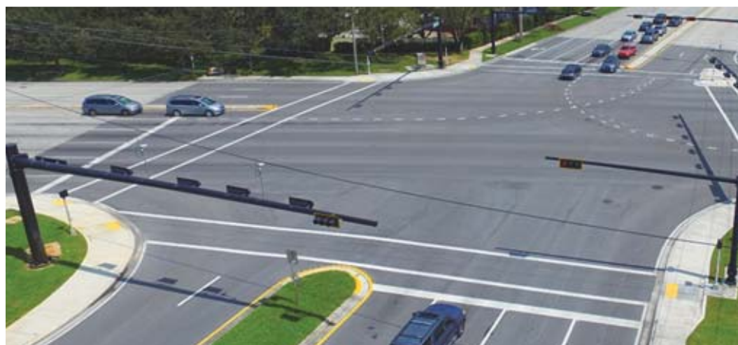
Flamingo Rd and Broward Blvd. Supplementary traffic signal heads were installed on the back of the arm. This strategy helps with the visibility of signal heads that may be blocked by long arms at super elevated or skewed intersections when approaching these.
