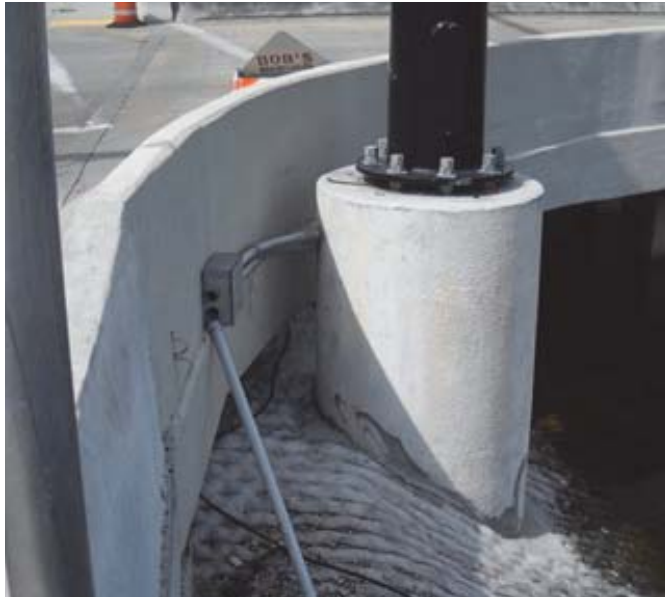
Broward Blvd. and Nob Hill Road. Concrete foundation designed and poured within the slope of the Old Plantation Water Control District due to the lack of space in front of the barrier wall.
