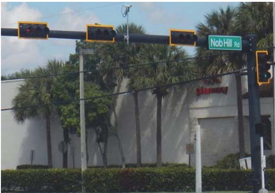
Broward Blvd. and Nob Hill Rd. Traffic signal heads were installed on the upright of the mast arm assembly. When primary signal heads are installed on uprights instead of the arms, the stresses on the arm are reduced. This is a great way to help balance the load for long mast arms at busy intersections with multiple travel lanes.
